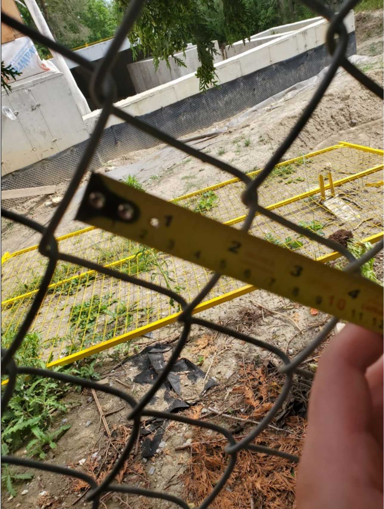
Attachment 2: Municipal Standards Officer's Photo - 7 Cicada Court - Existing pool enclosure. – Existing Metal Fence Opening
