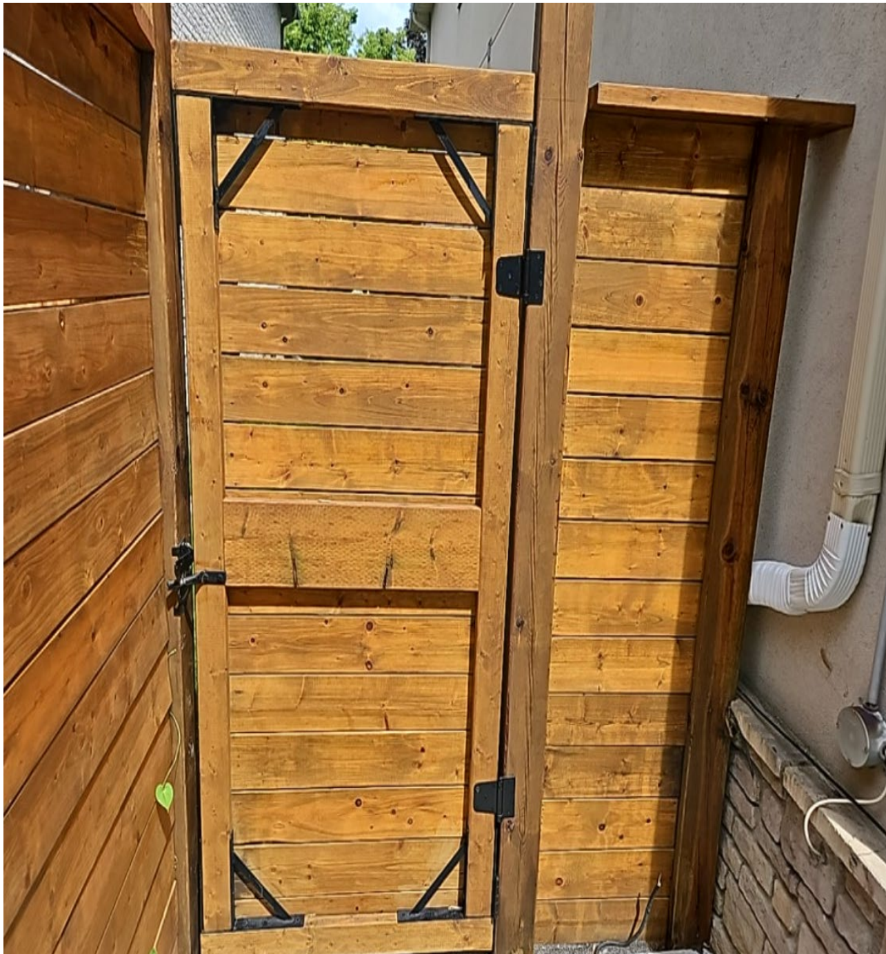
Attachment 2: Municipal Standards Officer's Photo - 115 Munro Boulevard - Existing Pool Enclosure. – Pool Gate - Side Yard
