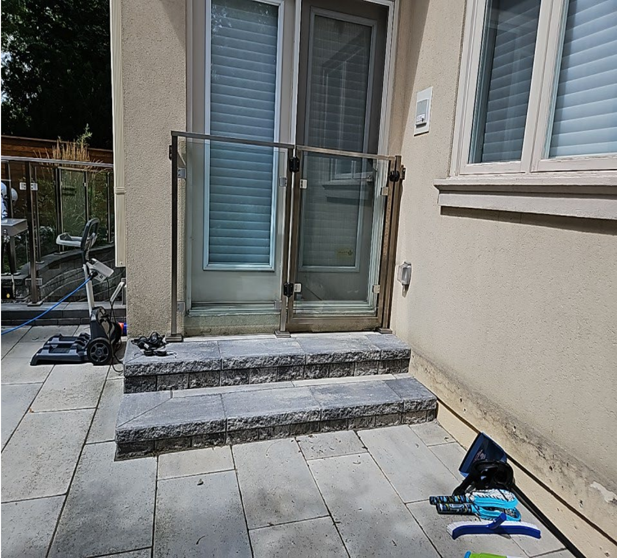
Attachment 3: Municipal Standards Officer's Photo - 115 Munro Boulevard - Existing Pool Enclosure - Juliet Balcony.
