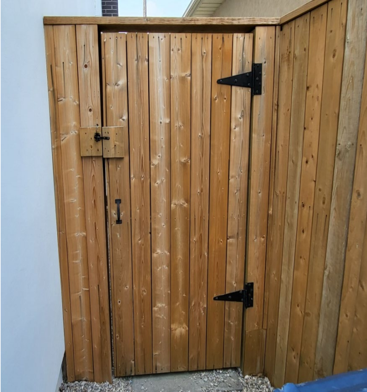
Attachment 6: Municipal Standards Officer's Photo – 311 Patricia Avenue - Existing pool Enclosure. – Side Yard Gate.
