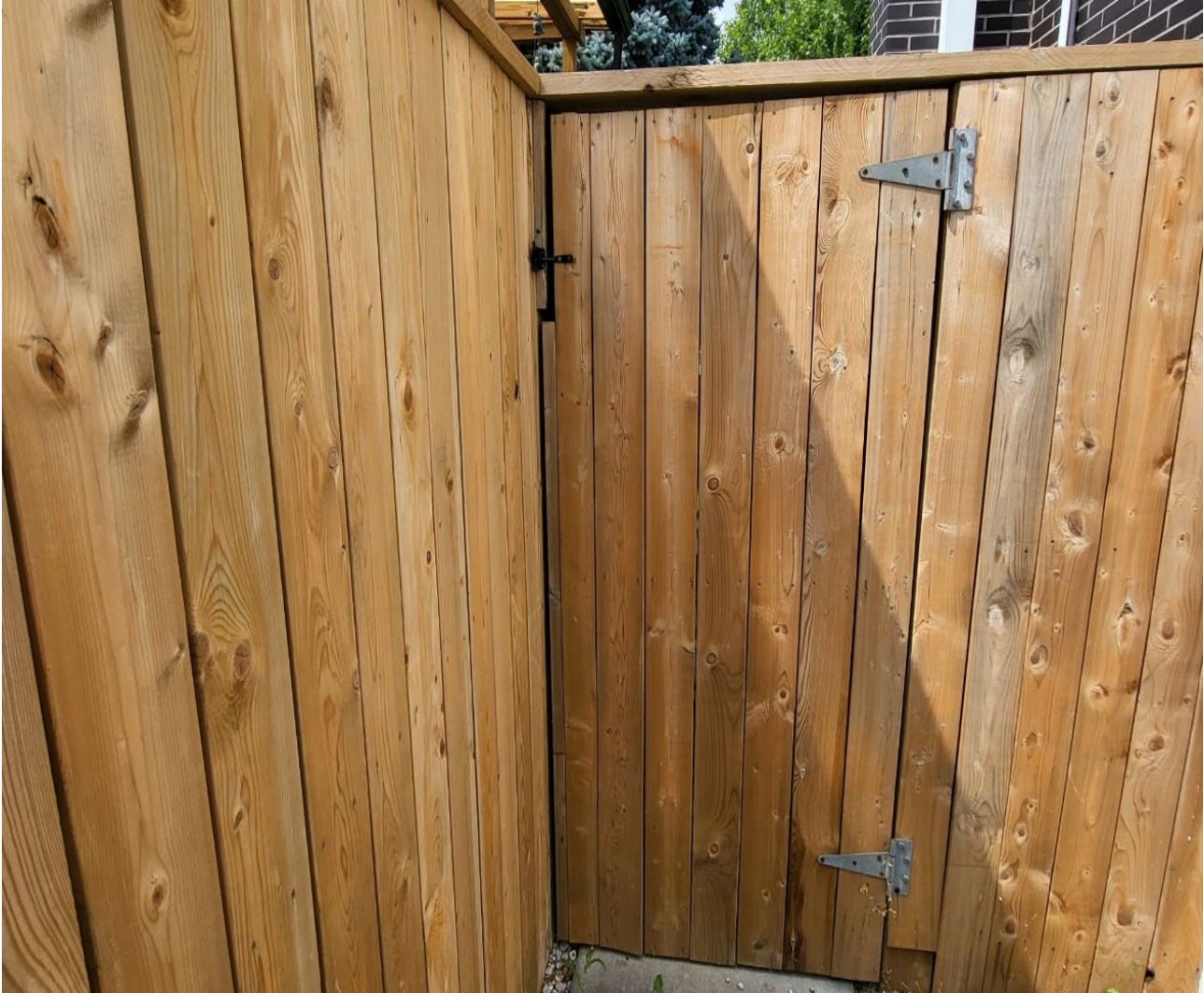
Attachment 3: Municipal Standards Officer's Photo - 311 Patricia Avenue - Existing pool enclosure. - Side yard Gate.
