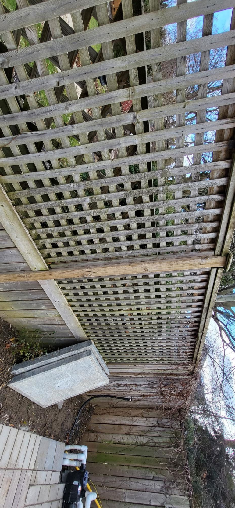
Attachment 5: Officers Photo – East side of the property viewing the inside fence of the pool enclosure of 335 Burnett Ave
