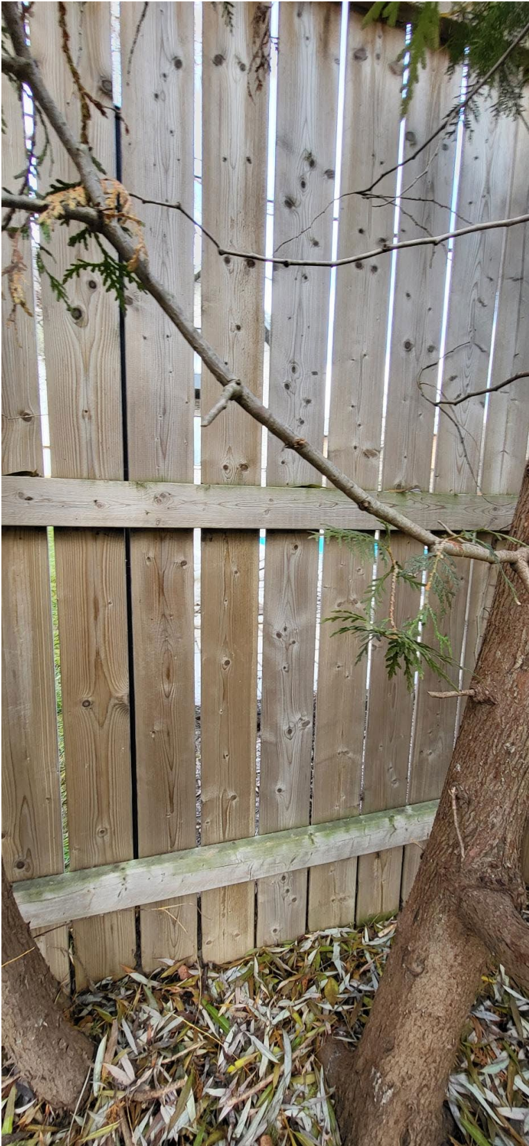
Attachment 4: Officers Photo – South side of the neighbours property viewing the outside of the pool enclosure of 335 Burnett Ave
