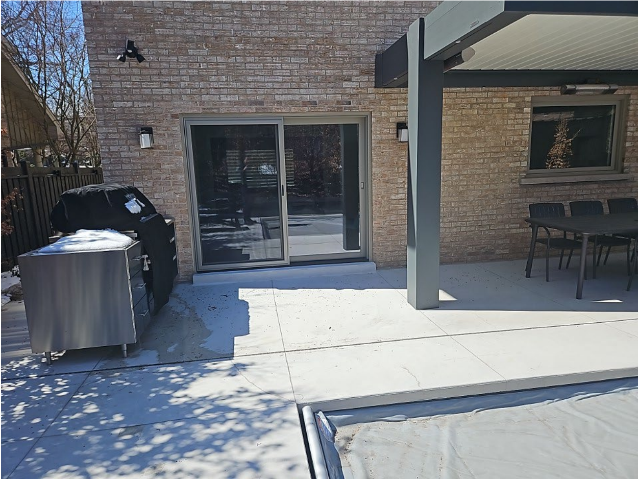
Attachment 3: Municipal Standards Officer's Photo - 51 Tanbark Cres - Rear Yard dwelling access to pool area.
