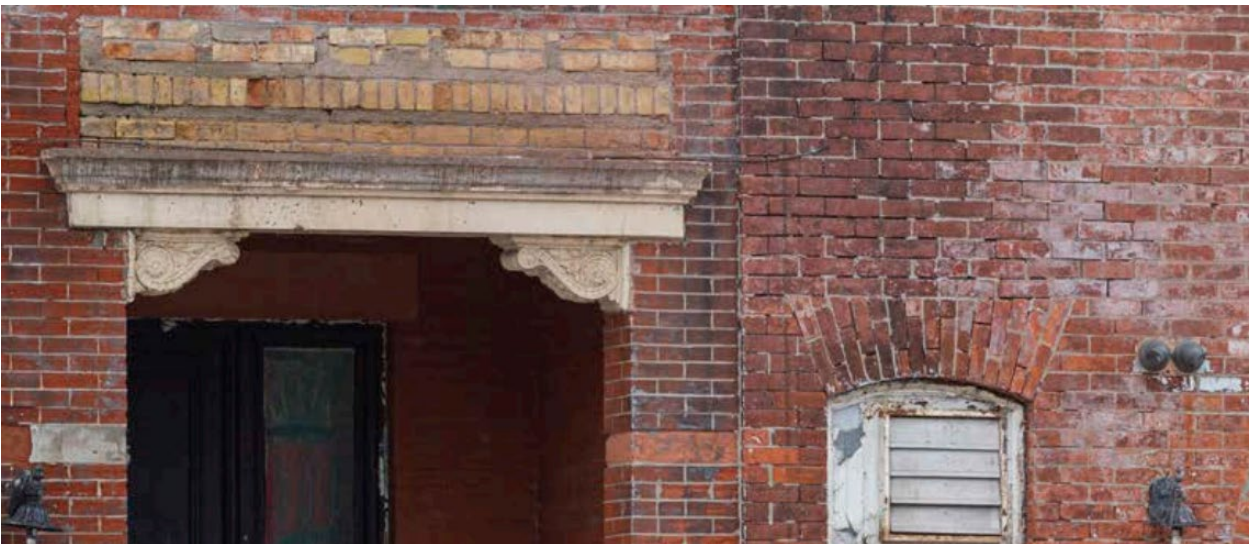
4. Examples of damage to masonry (Giaino Architects Inc. Reconstruction Plan, Dec 8, 2023)
