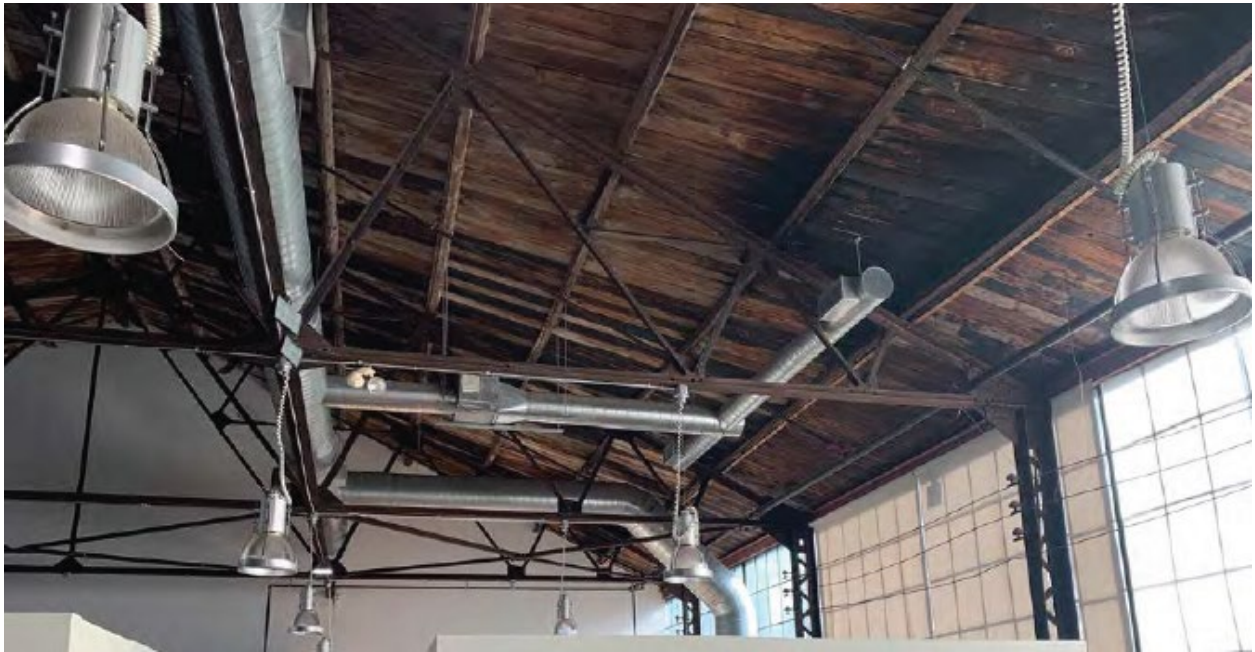
Figure 16. Interior view of the A. R. Williams Machinery Company Warehouse showing steel truss ceiling, 2023 (Heritage Impact Assessment, E.R.A. Architecture)
