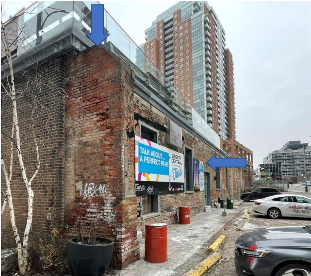
Figure 14. Portion of south and east elevations of the A. R. Williams Machinery Company Warehouse showing remnant party wall of the former Central Prison building indicated by blue arrows, 2024 (Heritage Planning)
