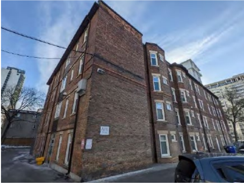
View of the northwest elevation at 36 Maitland Street (LHC Heritage Planning & Archaeology Inc, 2023).
