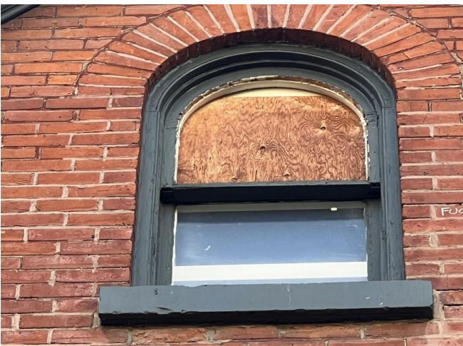
Windows in poor condition at 99-101 Maitland Street. RJC, 2023.
