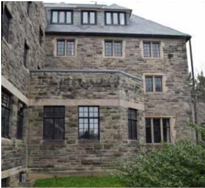
Figure 8. Partial view of the east elevation of the Convent (north) Wing, looking west, that shows the one-storey service component that is proposed to be demolished (ERA Architects Inc., May 2022).
