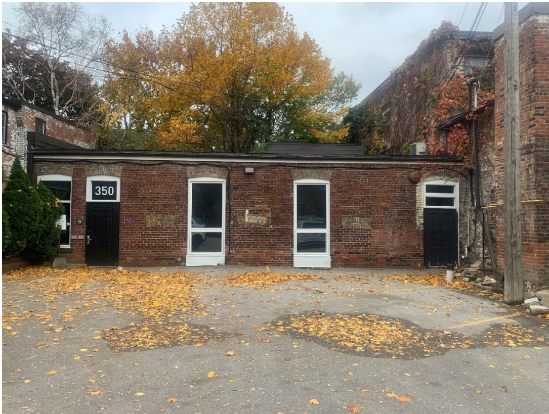
Image 22: Current photograph of the Mixing building, east elevation from the central courtyard. (Heritage Planning, 2024)
