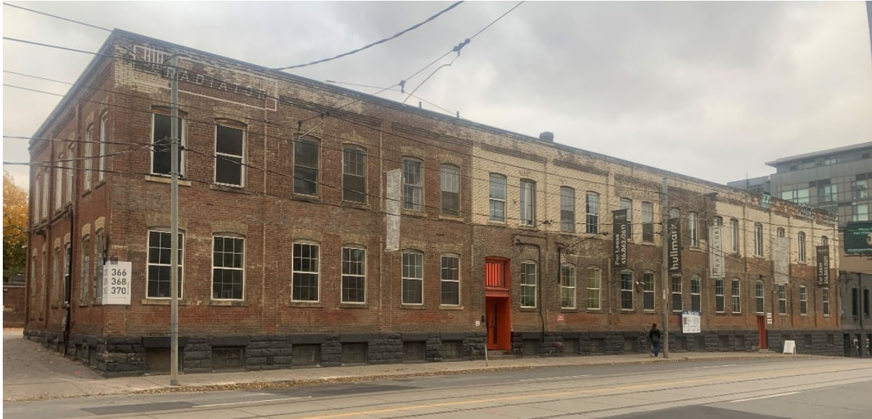
360 Dufferin Street, east elevation, showing the driveway providing access to the central courtyard, at left (Heritage Planning, 2024)
