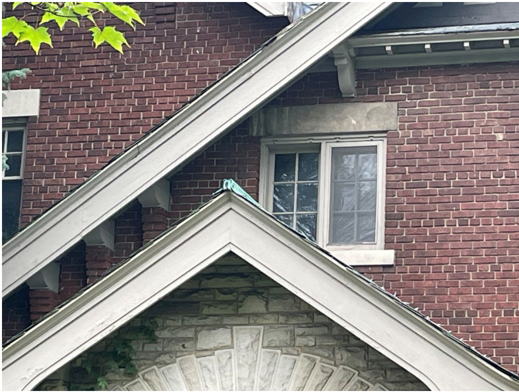
Figure 9: detail view showing an example of the brick corbelling and stone brackets below the eaves and the gable overhang detailing, 2024 (City of Toronto Heritage Planning)
