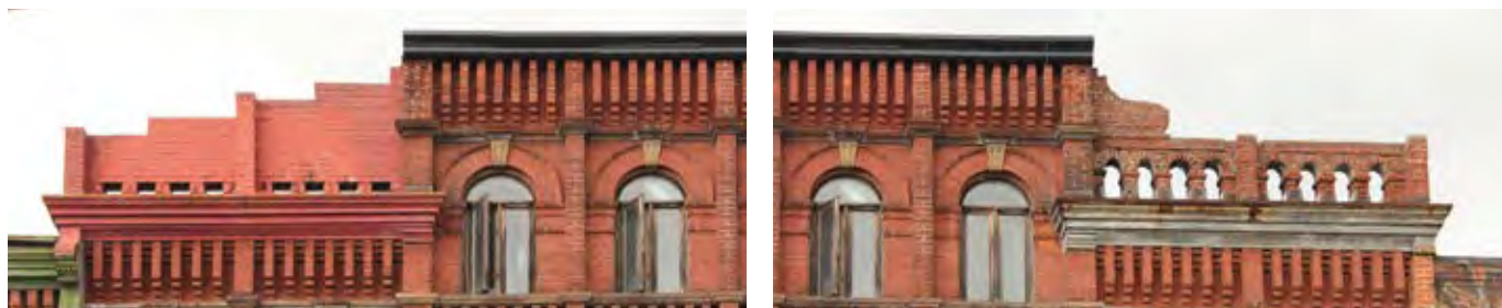
Figure 74: Detailed photo of the parapet at 660 and 664 Queen Street West that illustrates uneven repairs to deteriorated features but could be an opportunity for future restoration.
