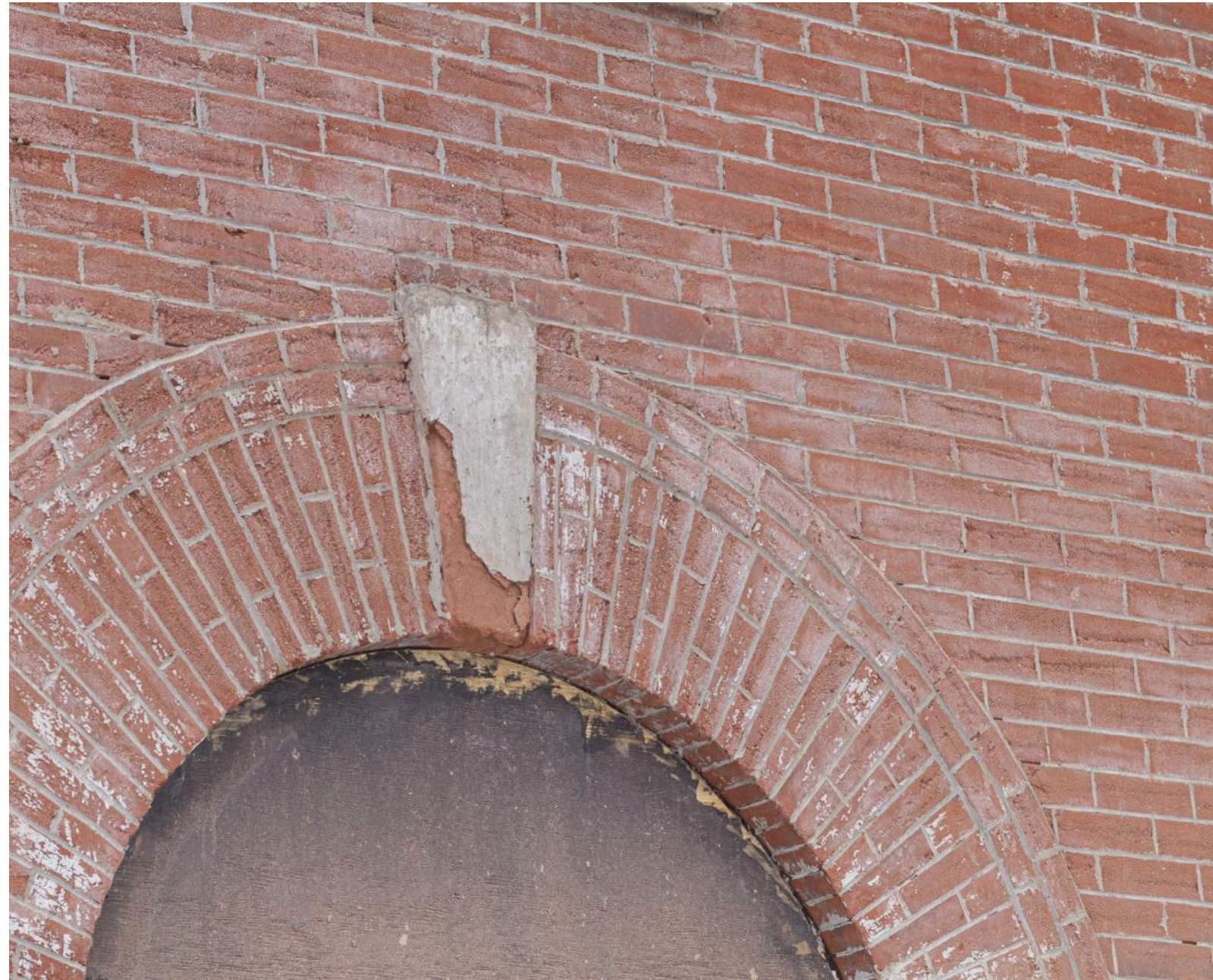
Field-view showing overcut joints, repointing with concrete, loss of stone and brick faces.
