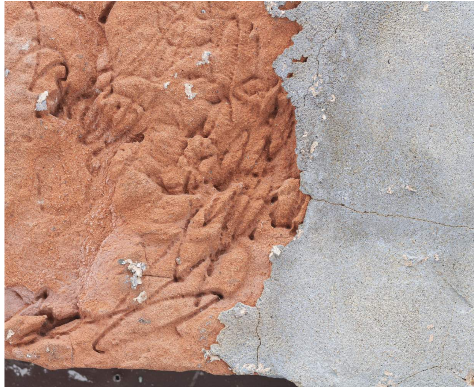
Visible gouging on stone due to power washing
