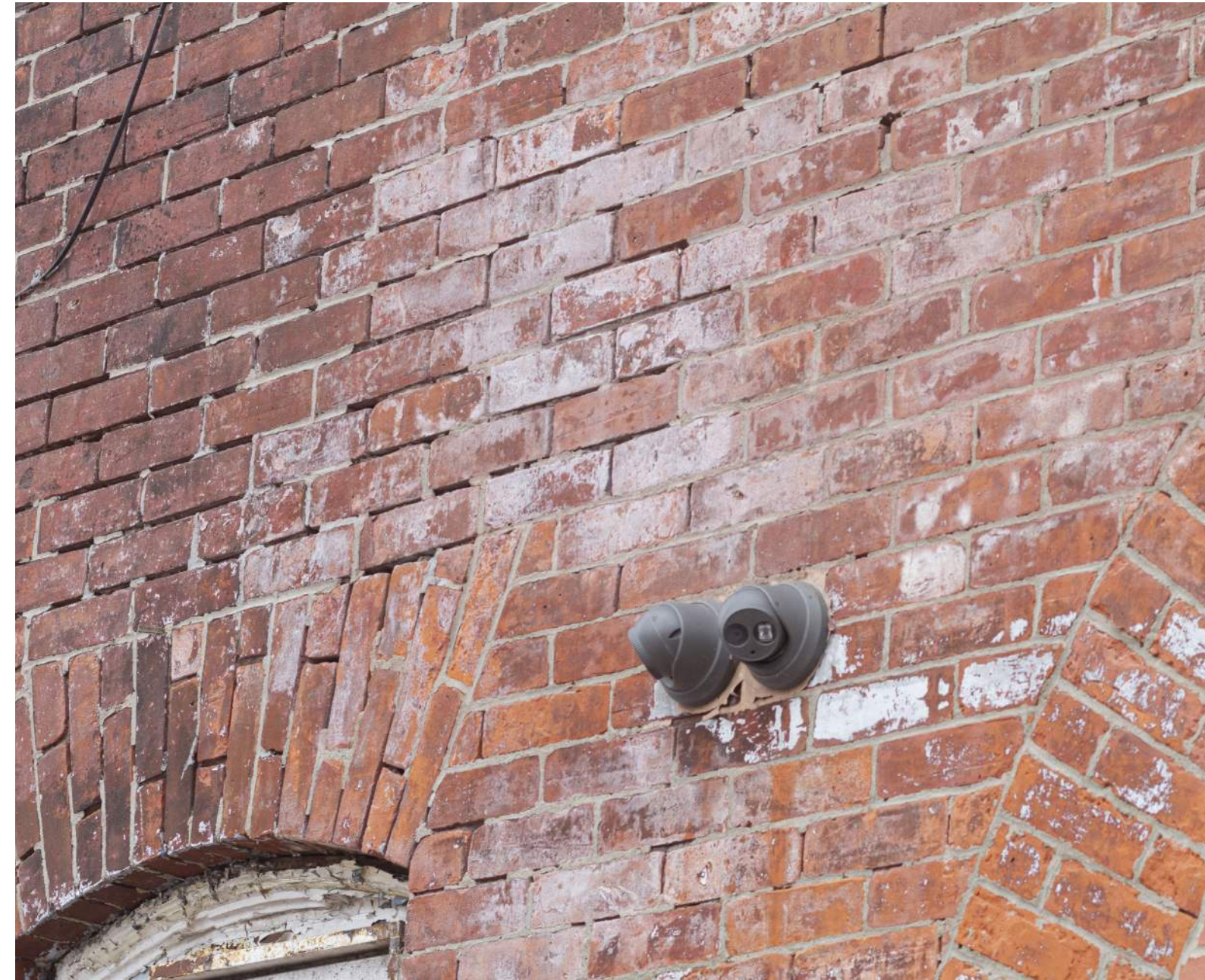
Poorly cut out brick joints, and loss of brick faces
