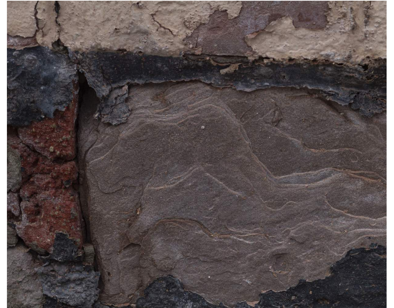
Stone delamination due to weathering
