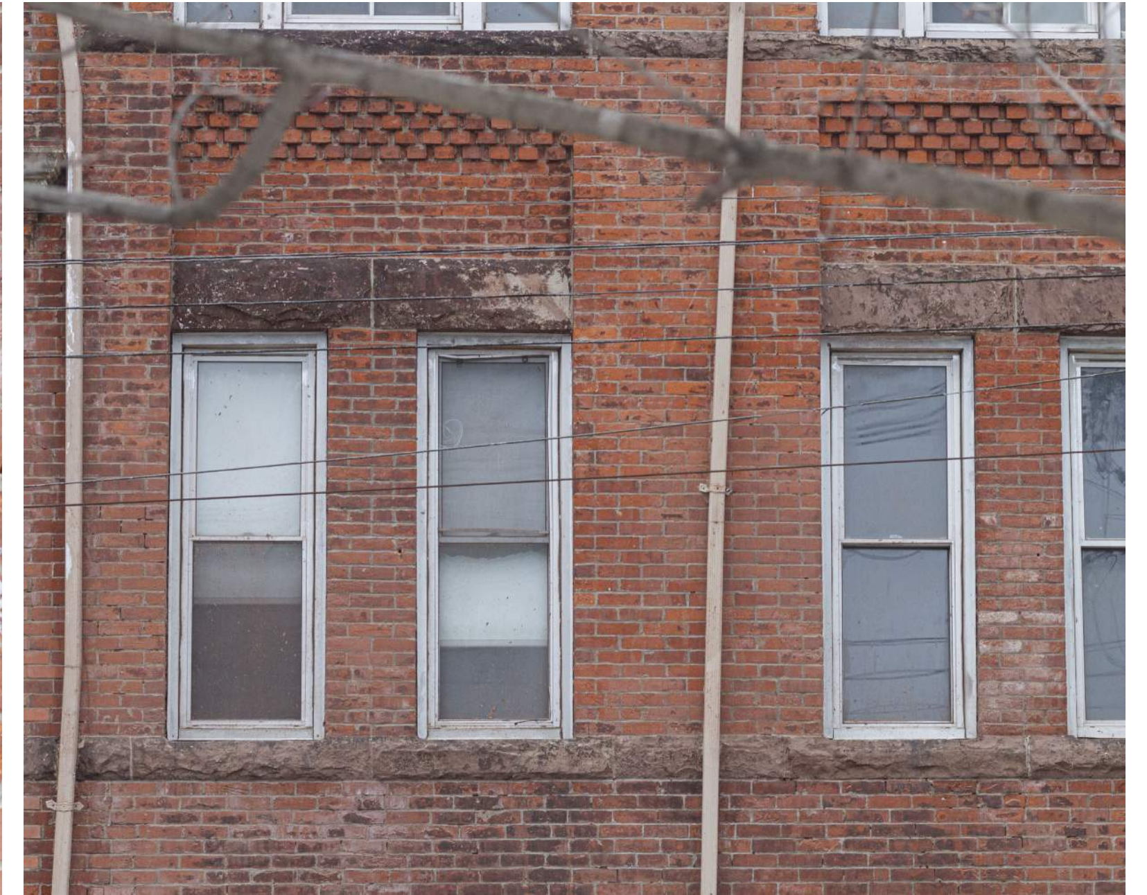
Poorly cut out brick joints, and loss of brick faces
