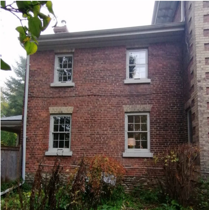
6. View of the south elevation of the rear ell showing 6 over 6 windows with buff brick voussoirs (Heritage Planning, 2023).
