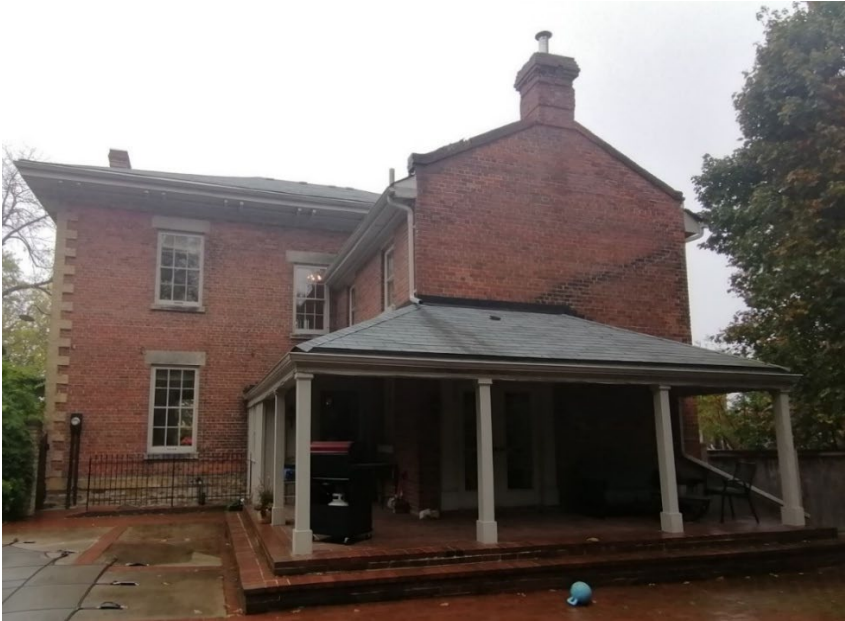
5. View of 1 Heritage Place looking northeast, showing the rear (west) elevation of the main structure and the north and east (rear) elevations of the rear ell. Note the brick parapet and chimney on the rear elevation of the rear ell and ghosting of rear lean to (Heritage Planning, 2023).
