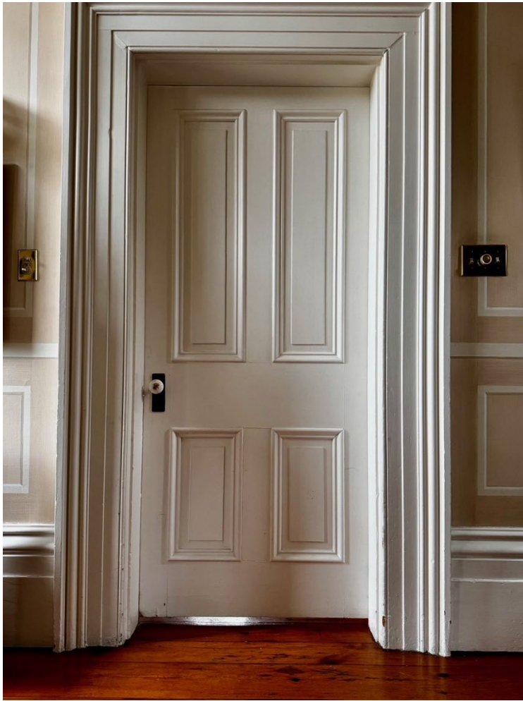
Figure 13 Interior image showing first floor millwork including baseboards, door trim and raised-paneled door (Heritage Planning, 2023).
