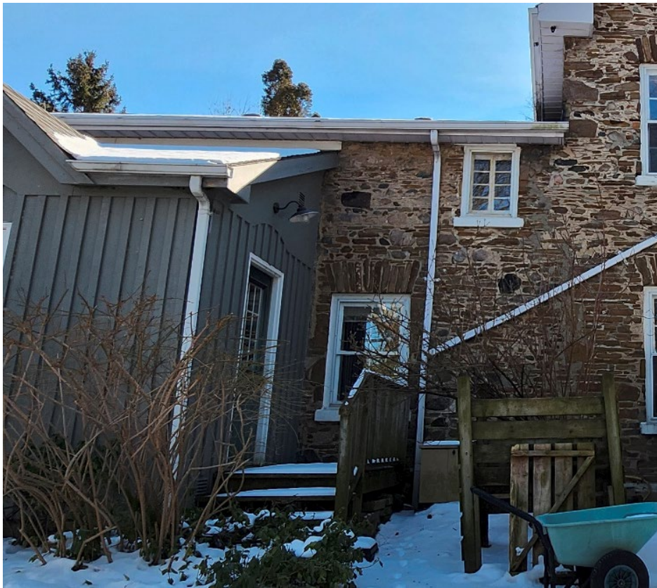
Figure 24. Detail of the two windows in the rear (north) wall of the rear kitchen wing (Heritage Planning, 2024)
