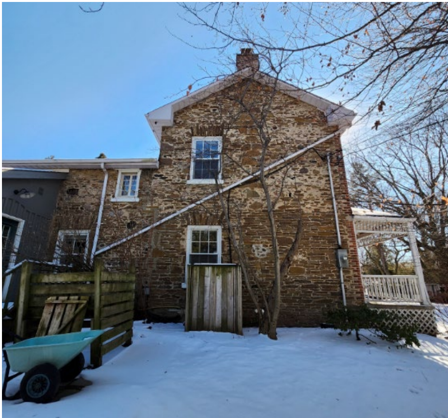
Figure 19. Detail of the side (north) elevation of the main house illustrating the windows and Humberstone (Heritage Planning, 2024)
