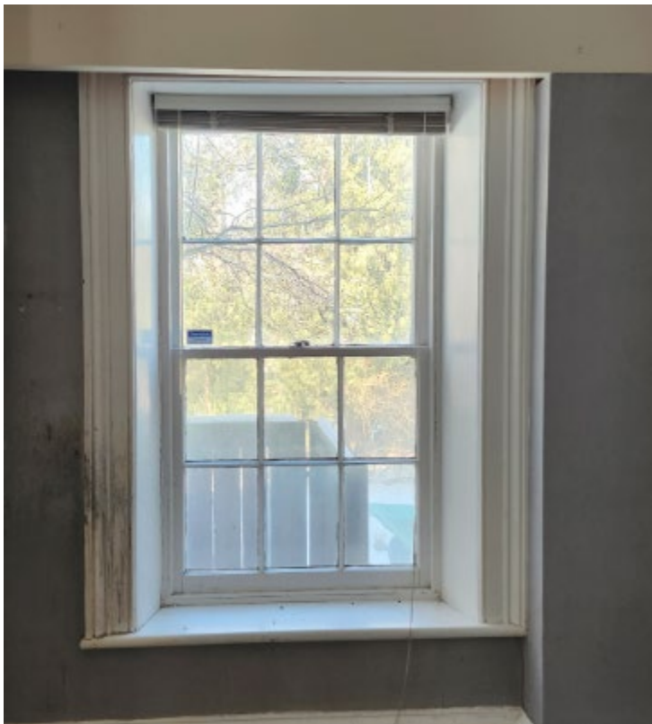
Figure 25. Detail of the casement of the window in the first storey of the side (north) wall of the main house (Heritage Planning, 2024)
