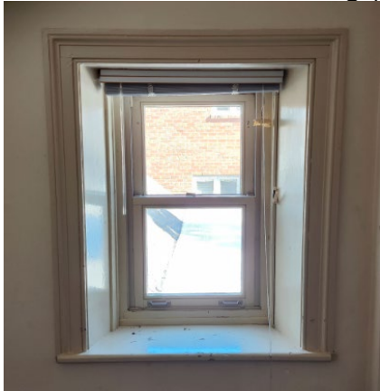
Figure 28. Detail of the casement of the window in the second storey of the side (east) wall of the rear kitchen wing (Heritage Planning, 2024)
