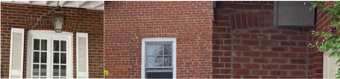
13. Detail comparison of the jack arch brick voussoirs on the original portion of the subject property (at far left) and the varied segmental arch brick voussoirs on the rear wing (Heritage Planning, 2023).
