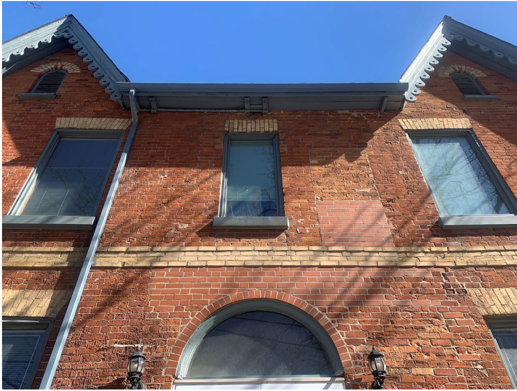
Figure 10. Detail of west elevation at 115 Berkeley Street showing an infilled opening at the second storey and differentiation of brickwork around the main entrance (Heritage Planning, 2024)
