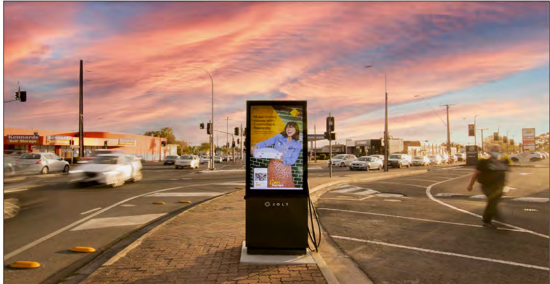
FIGURE 1: FREE-STANDING JOLT ELECTRIC VEHICLE (EV) CHARGING STATION (THIRD PARTY GROUND SIGN) WITH INTEGRATED ELECTRONIC SIGN FACE DISPLAYING ELECTRONIC STATIC SIGN COPY
