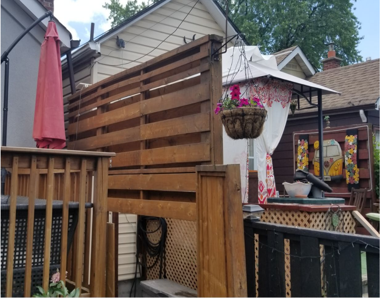
Attachment 4 Municipal Standards Officer's Photo 28 Byng Avenue –Rear Yard – South Side Fence
