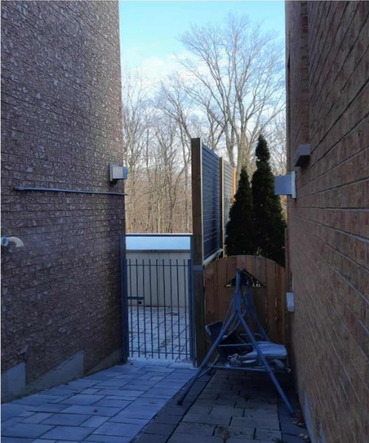
Attachment 2: Municipal Standards Officer's Photo - 70 Falaise Road - Rear Yard
