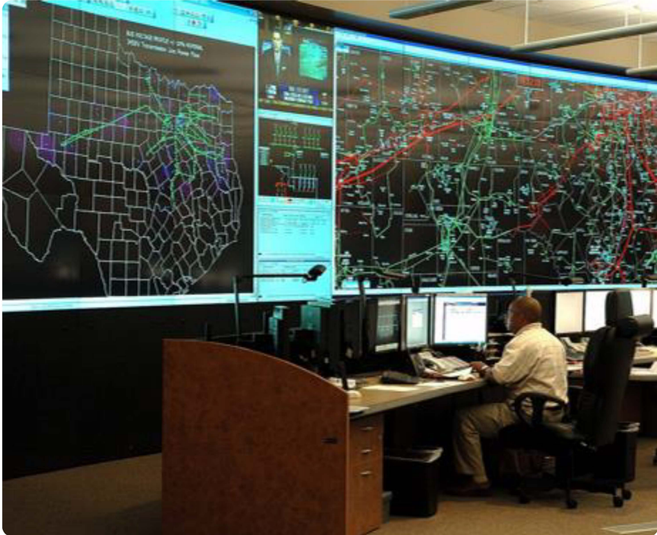
Oncor, an electricity transmission and distribution company (an OMERS Infrastructure investment) established a System Resiliency Plan focused on withstanding and rapidly recovering from extreme weather and other events
