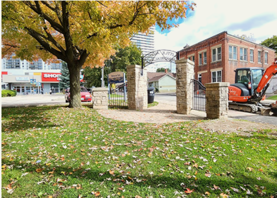
Figure 60: The revitalized entry gate (2009) gives the park identity, but doesn't connect to a path network, limiting its accessibility and usefulness as a gateway.
