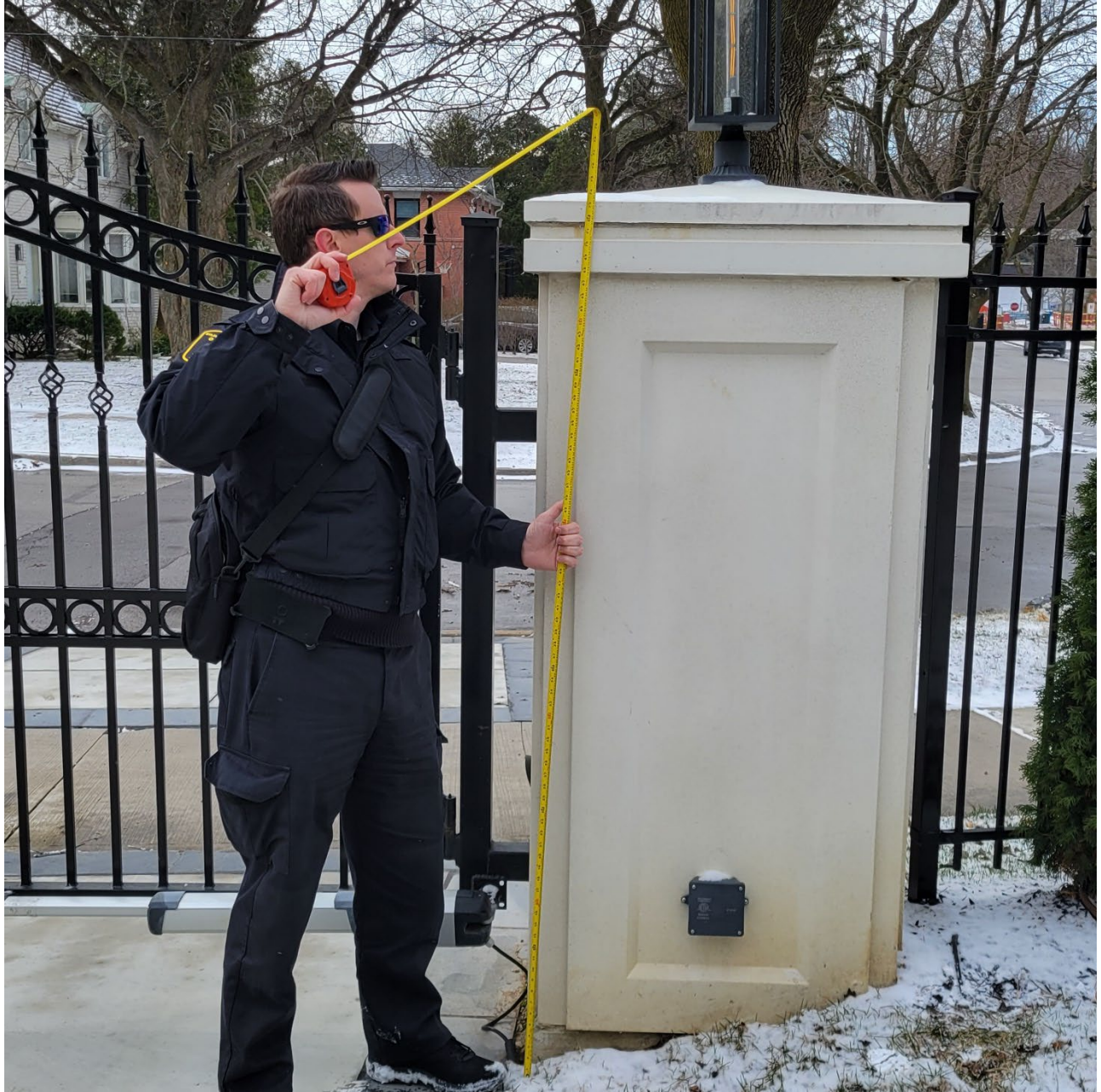
Attachment 10: Photograph depicting existing height of precast concrete columns at 1.86 metres. Maximum permitted height for any component of the fence is 1.2 metres.
