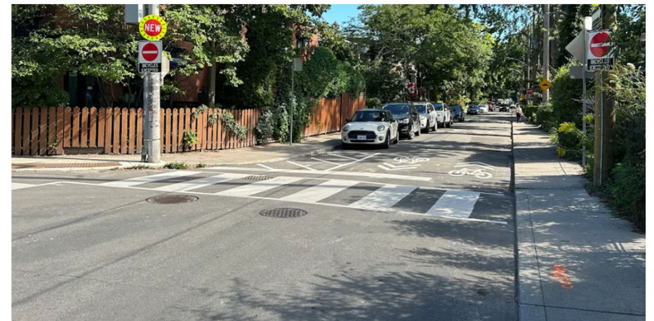
Macdonell Avenue and Rideau Avenue where a crosswalk was marked in advance of ramp construction
