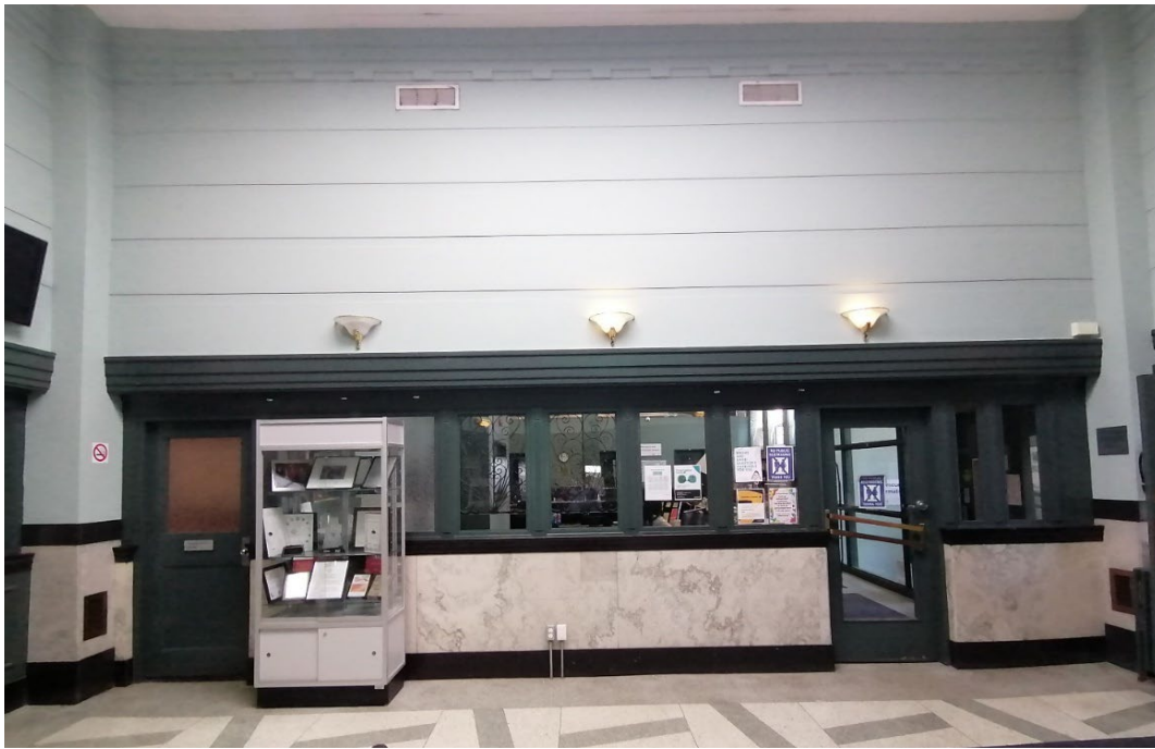
Figure 11 Interior image of the postal hall looking east showing original doors, plasterwork, terrazzo floors, marble dado, and wicket openings (Heritage Planning, 2024).
