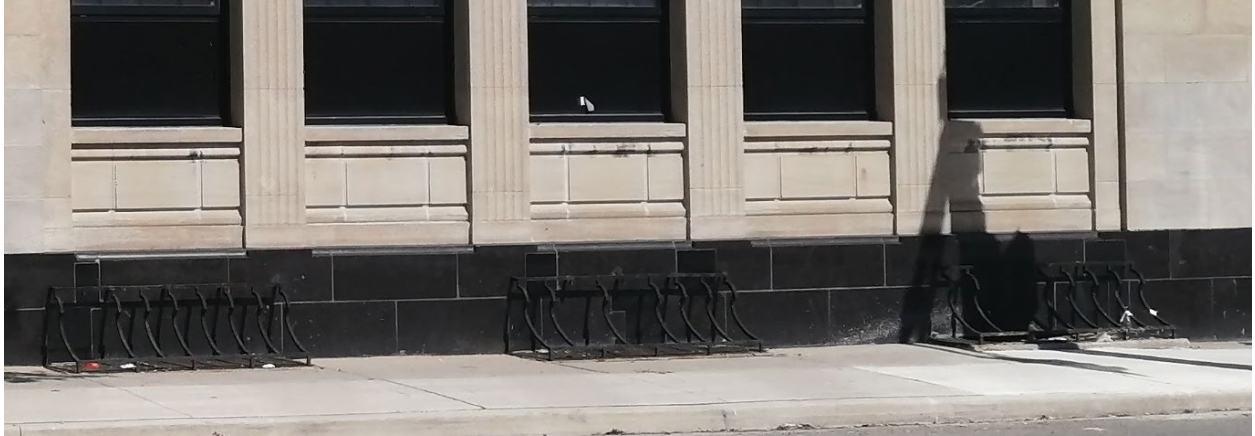
Figure 6 Detail of the blind balustrades and iron basement light well grilles on the west elevation of the 1935 structure's main wing (Heritage Planning, 2024).
