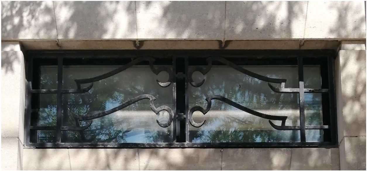
Figure 5 Detail of the iron transom grille on the west elevation of the 1935 structure's rear wing (Heritage Planning, 2024).
