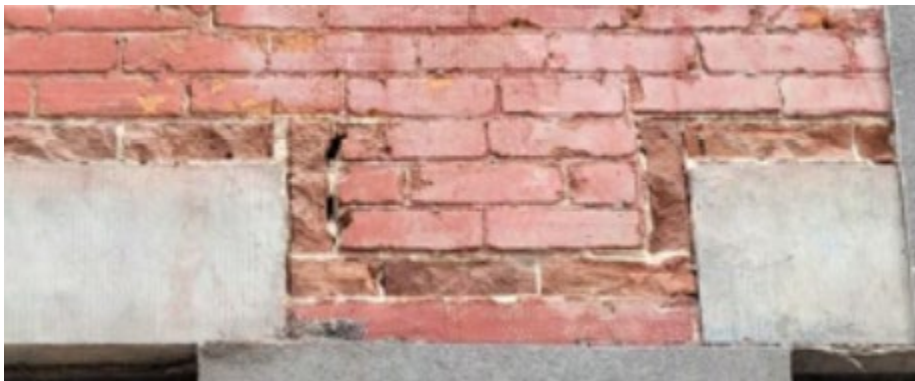
Extracts from photographs showing damaged brick at various testing locations at the building facades of the Margaret Grimmon Houses at 357-359 Richmond Street West. (Source: HIA dated March 5, 2025 from GBCA Architects and RJC Engineers)
