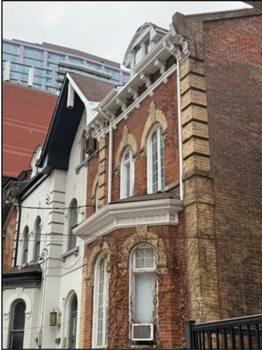
Figure 24. 344 Jarvis Street, showing primary facade configuration with bay window, brackets, and quoins (Alex Corey Heritage Consulting, 2025).
