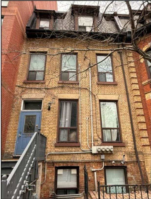
Figure 16. Detail of the primary (east) facade of 336 Jarvis Street (Alex Corey Heritage Consulting, 2025).
