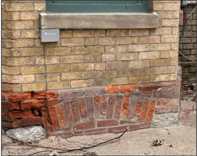
Figure 22. Foundation details at 209 Jarvis Street showing red brick above stone foundation and bricked-in lower level window opening (Alex Corey Heritage Consulting, 2025).
