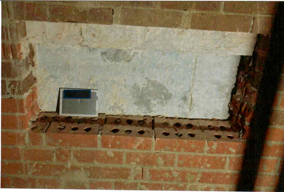
Figure 18 Investigation opening #5 in vent shaft.
