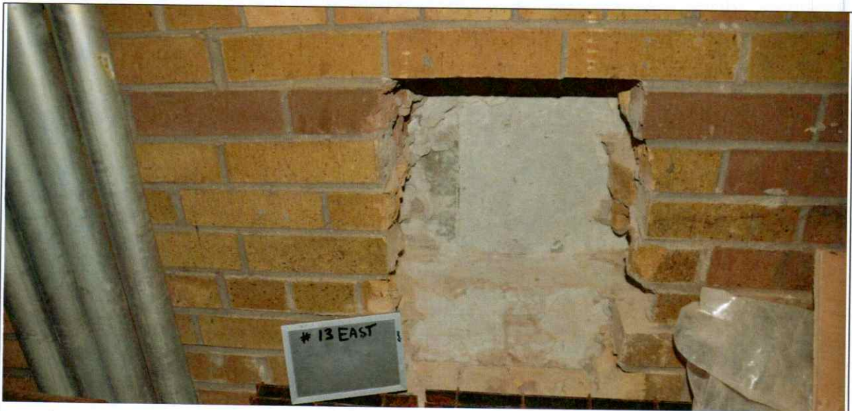
Figure 34 Investigation opening #13 in vent shaft.
