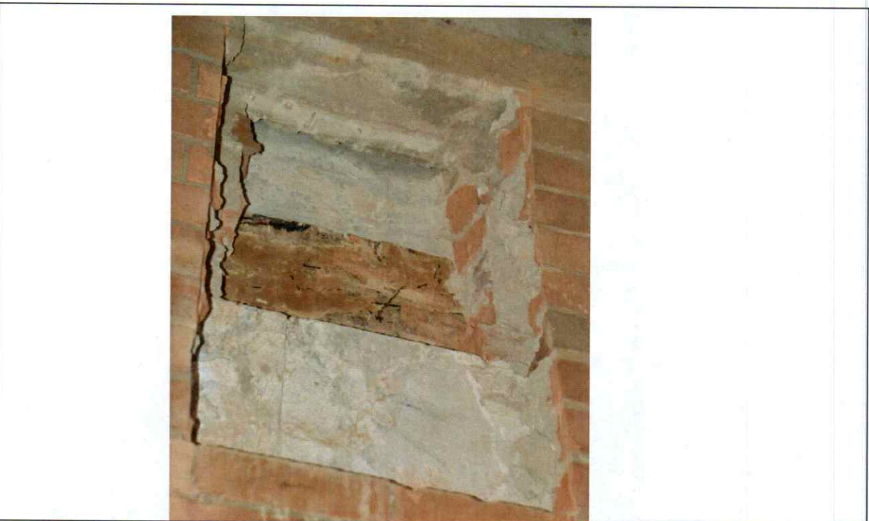
Figure 23 Investigation opening #7 Stone veneer is block bonded with brick backup. No ties were found.
