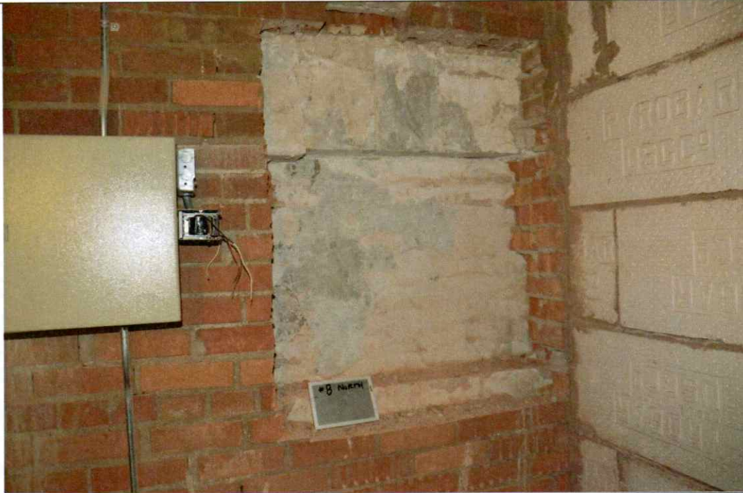
Figure 24 Investigation opening #8 in vent shaft.
