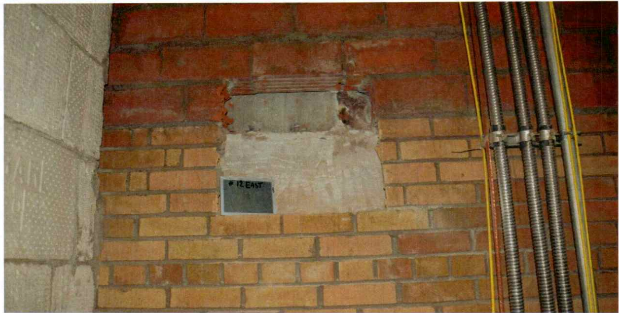
Figure 32 Investigation opening #12 in vent shaft.
