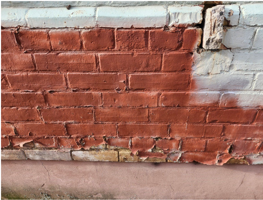
Figure 23. 29 Sussex Avenue showing the original buff brick in the side (east) elevation below the peeling paint (Heritage Planning, 2024)
