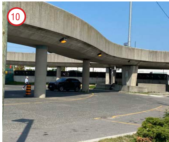
Figure 1.20 Existing Line 3 SRT Infrastructure
