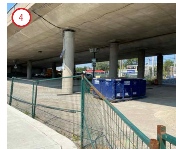
Figure 1.8 Lack of Lighting in the Underpass
