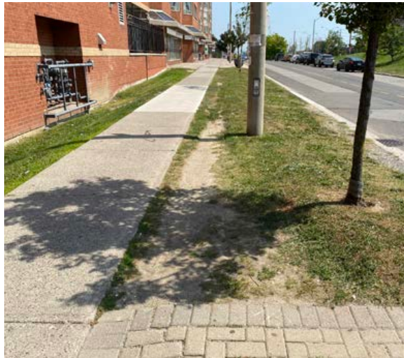
Figure A2.61 Existing Condition at Rainbow Village
