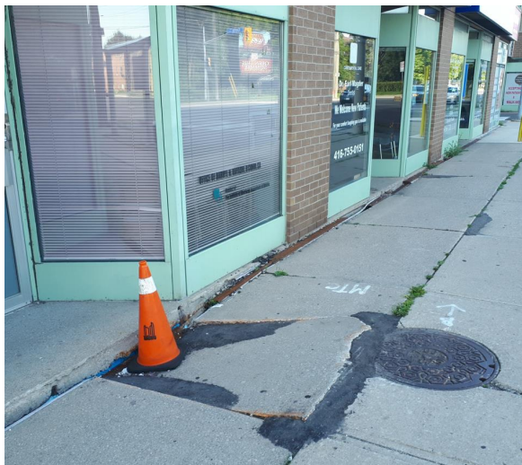
Permanent repairs required
