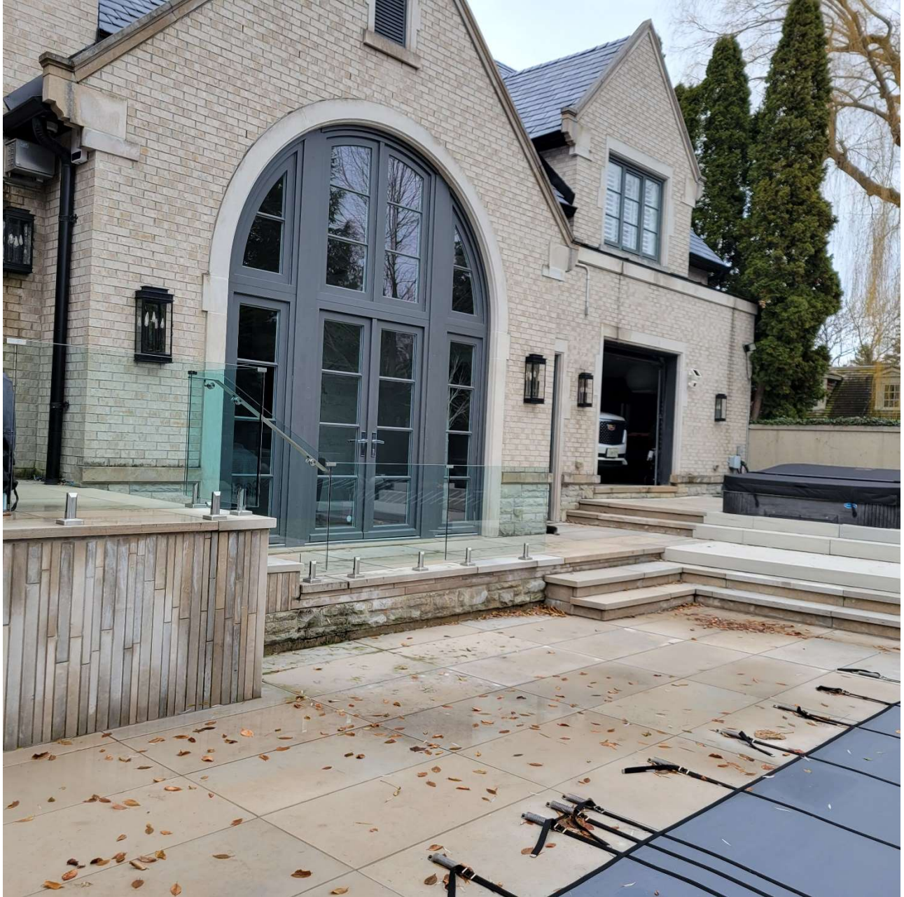
Attachment 7: Photograph depicting no self closing/self latching gate at bottom of stairs separating pool enclosure from direct access to the dwelling AND no self closing/self latching gate to restrict access from garage entry
