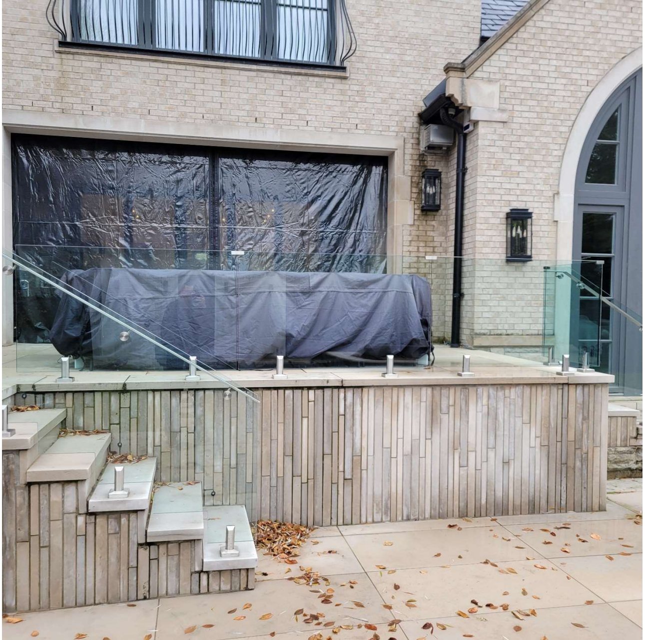
Attachment 6: Photograph depicting no self closing/self latching gate at bottom of stairs separating pool enclosure from direct access to the dwelling
