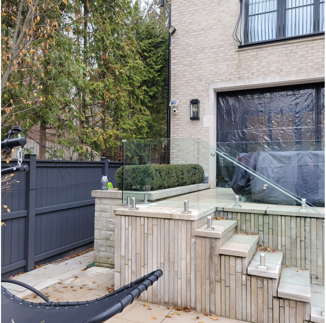
Attachment 5: Photograph depicting no self closing/self latching gate at top of stairs separating pool enclosure from direct access to the dwelling
