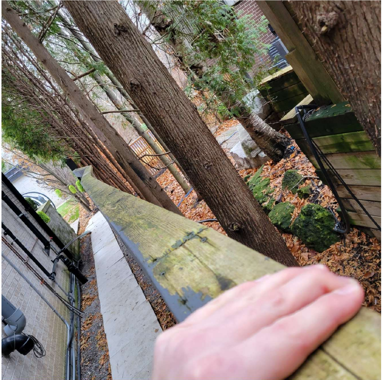
Attachment 13: Photograph depicting wooden perimeter pool enclosure fence located along west side yard. Fence is not maintained in a plumb or structurally sound condition.
