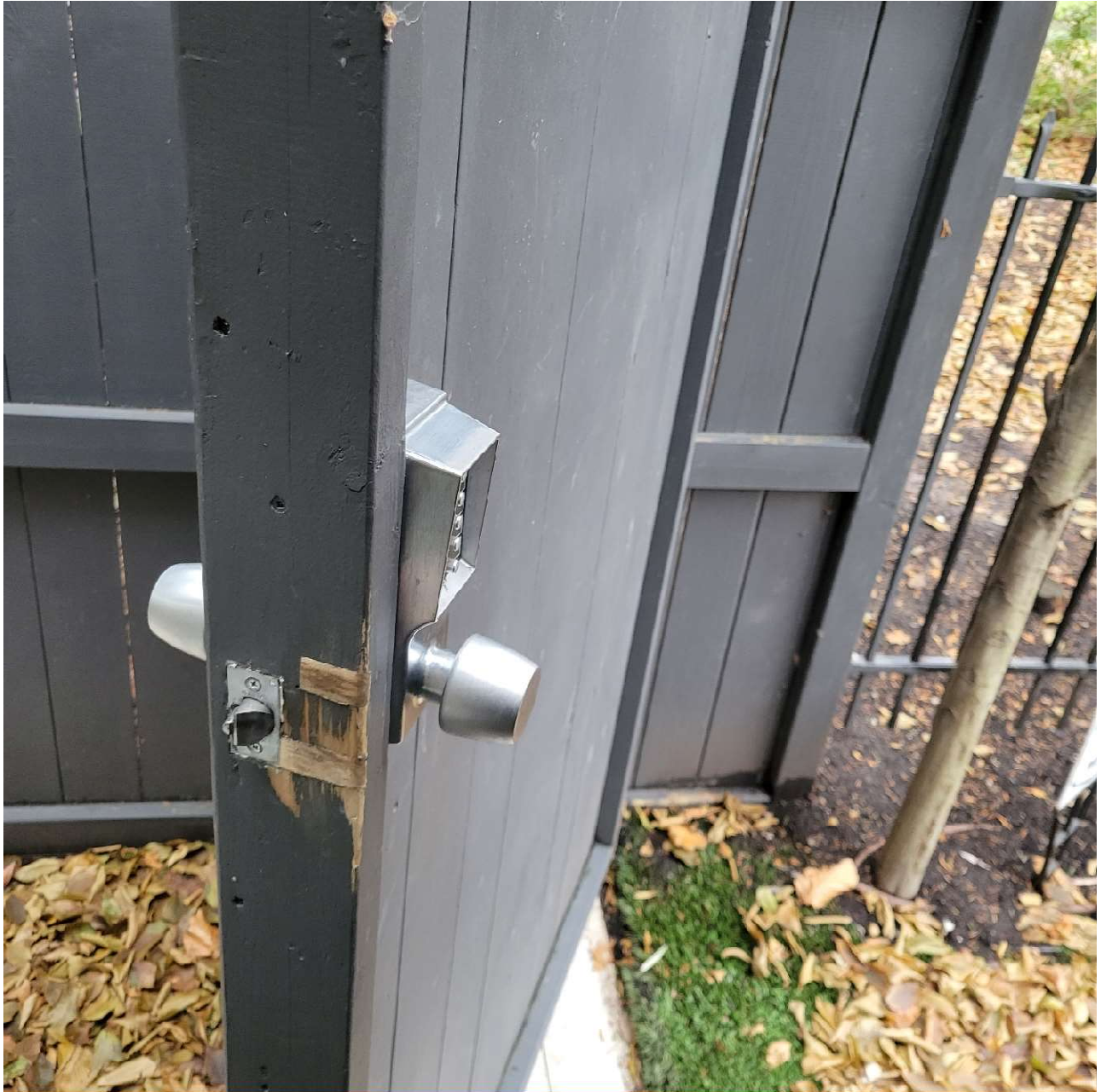
Attachment 11: Photograph depicting wooden gate, that forms part of the pool enclosure, located at the North West Side yard of property, gate is not self-closing
