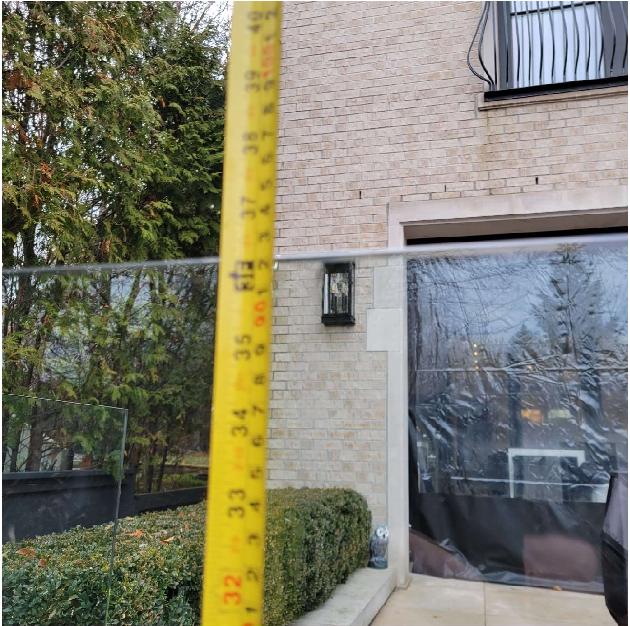
Attachment 8: Photograph depicting existing glass fence, of 0.92 metres in height. Minimum height for pool enclosure is 1.2m.
