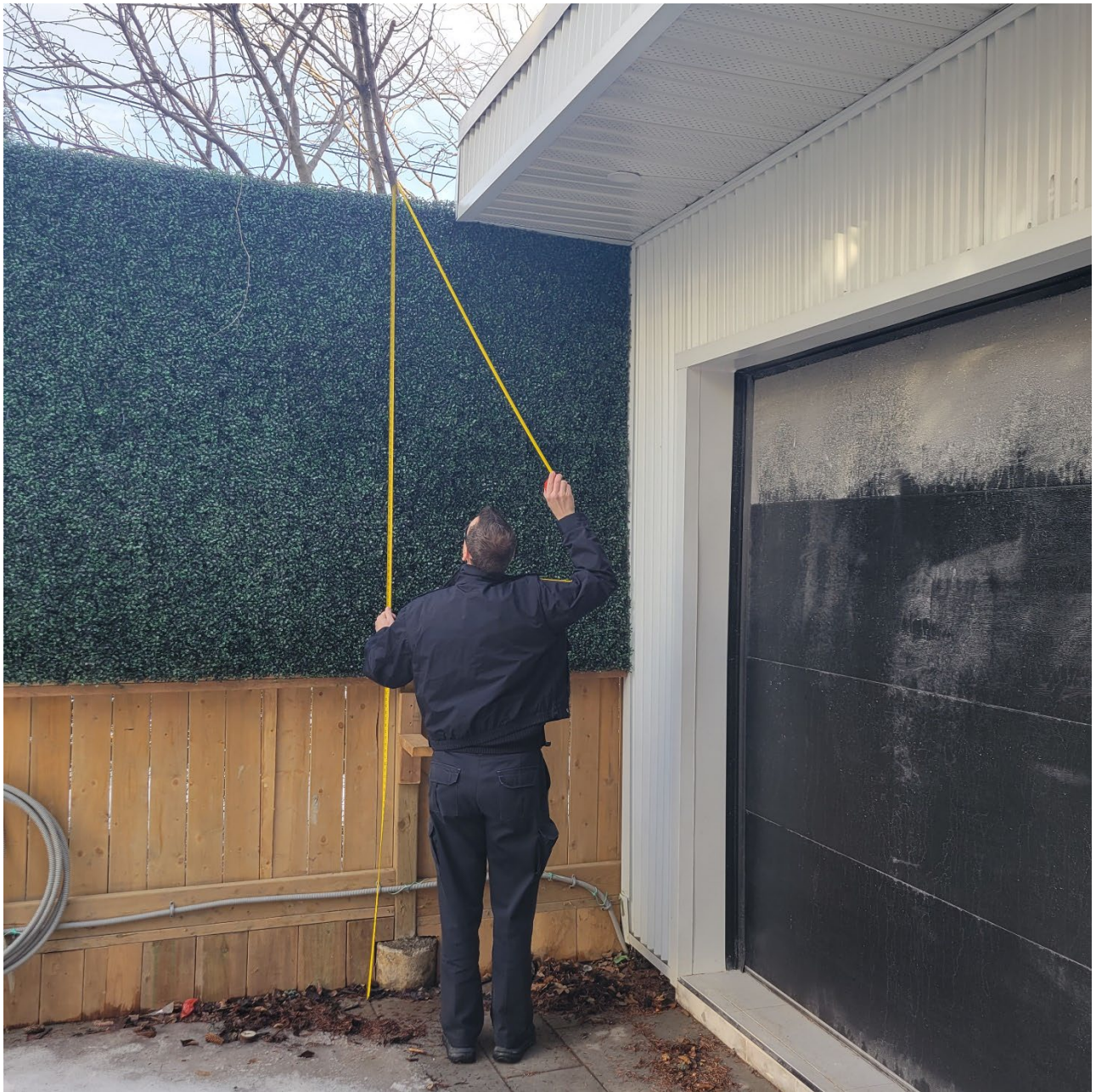
Attachment 11: Photograph depicting existing northern fence, of 3.14 metres in height. Maximum height for the fence is 2m.
