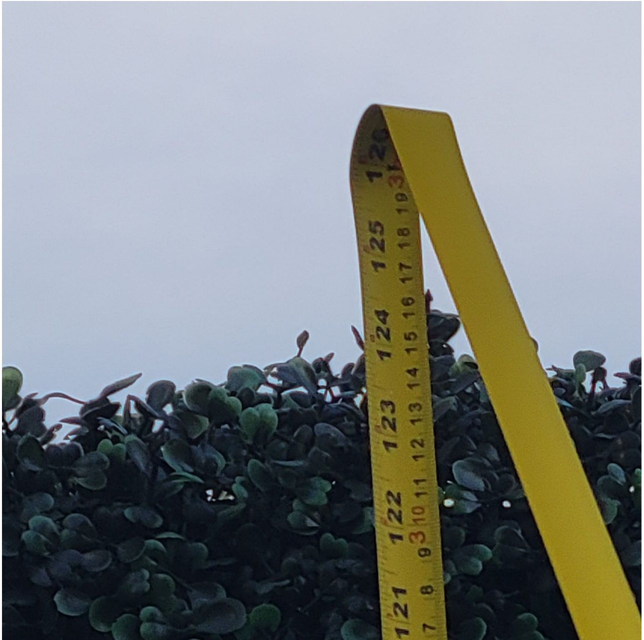
Attachment 10: Photograph depicting existing northern fence, of 3.14 metres in height. Maximum height for the fence is 2m.
