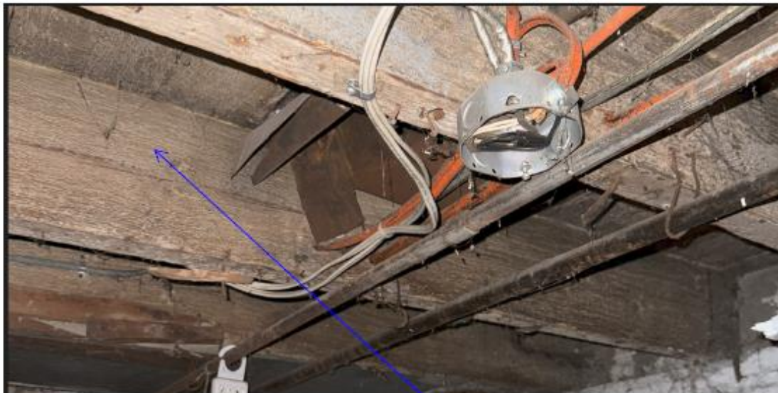
Mold on foundation Joist system
