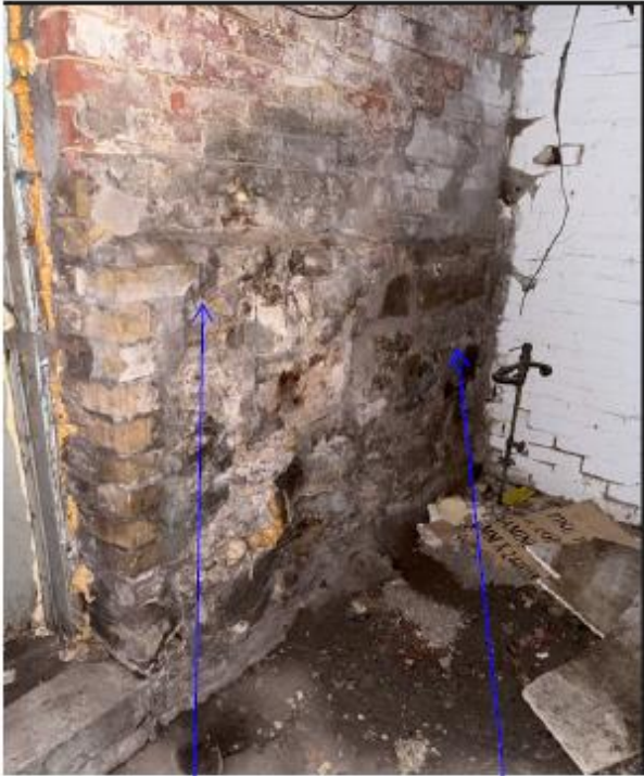
Foundation wall made of stone and brick . Visual Moisture
