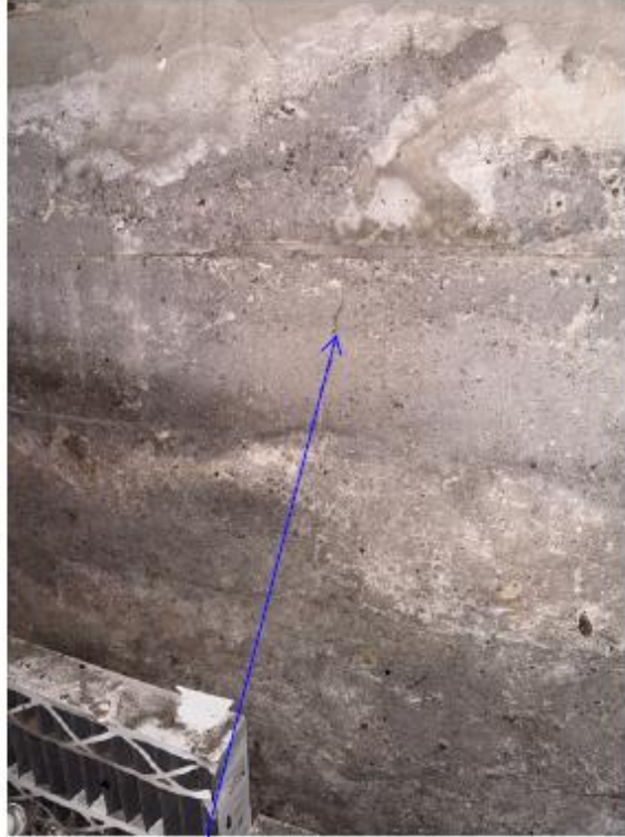
Concrete Wall cracke
