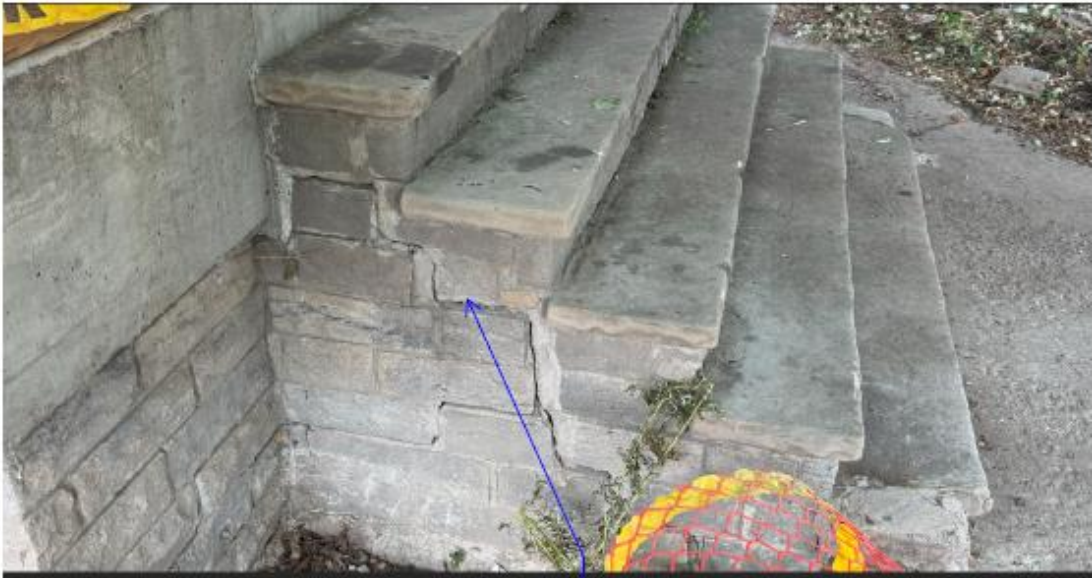
Crack Front Entrance stairs
