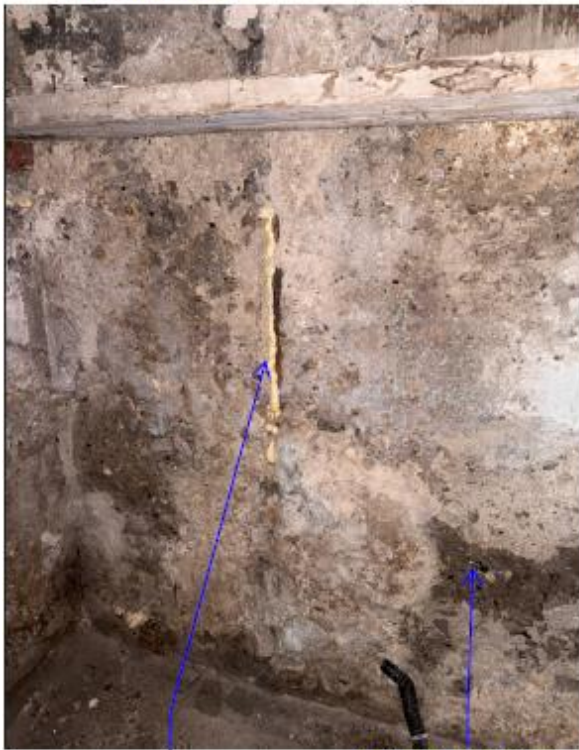
Foundation wall crack filled with foam
