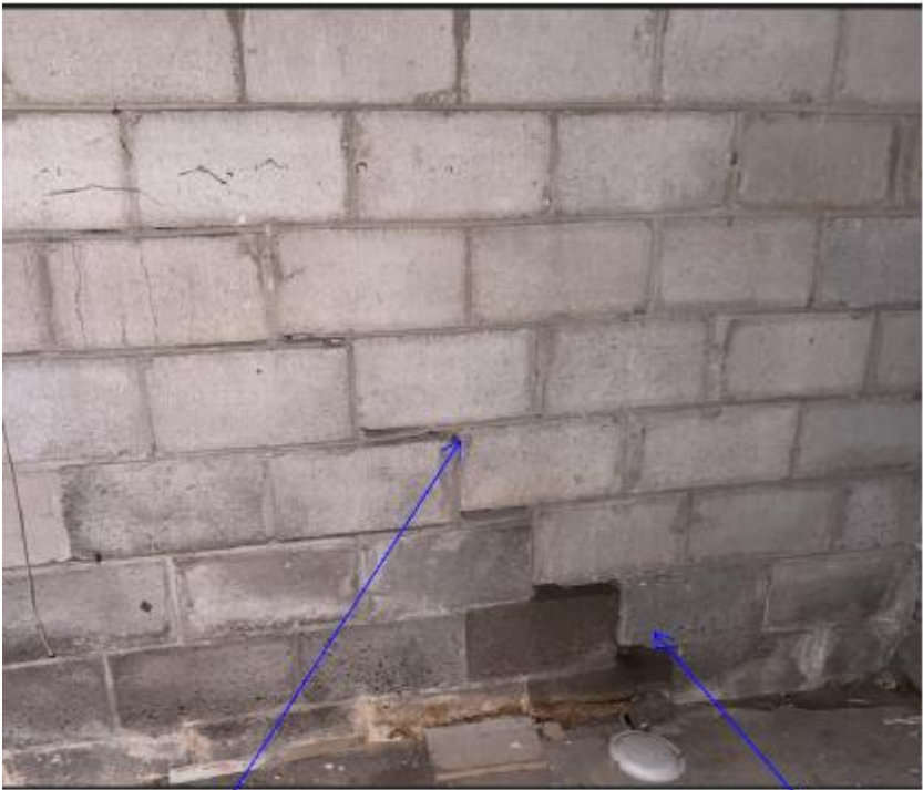
Concrete Block Foundation wall Shifted crack
