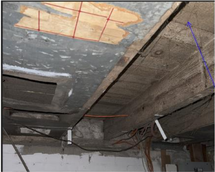
Mold on foundation Joist system
