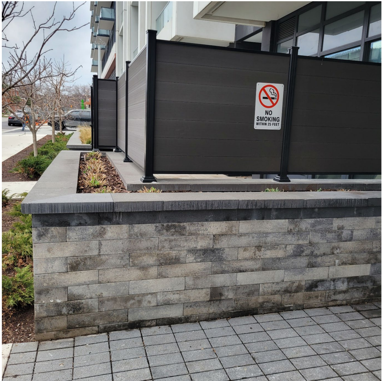
Attachment 4: Photograph depicting Fence on the west side of the building, flanking Sumach St, looking north, lower masonry and upper aluminum/composite fence (2.0m).
