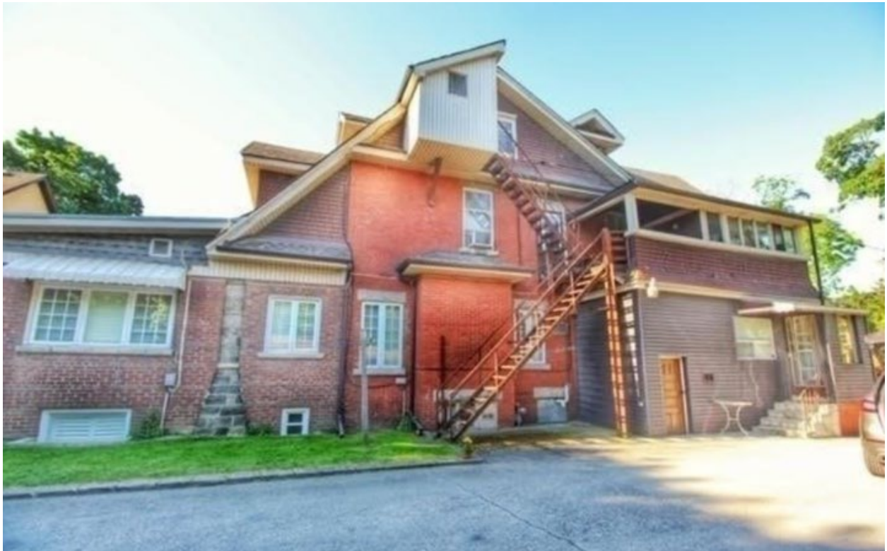
Figure 6: North (rear) elevation - historic verandah supports within the 1955 alterations (Royal LePage Signature Realty, Brokerage 2021)
