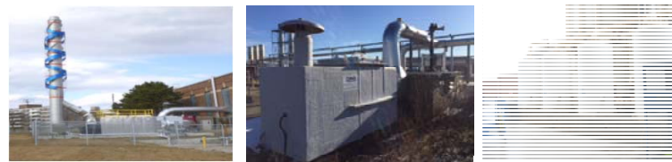
M building scrubber
