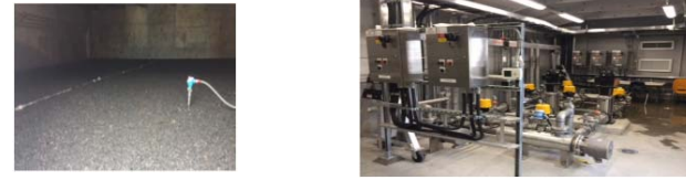
Biofilter bed at truck loading & biosolids storage silo building
