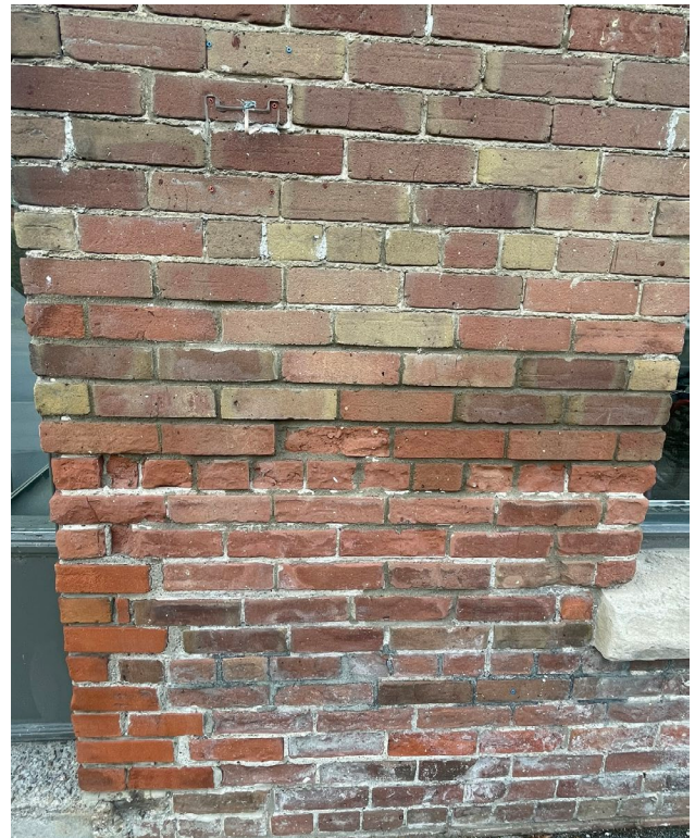
Fig. 5.4. North facade: example of brick condition at the building base showing brick replacement.
