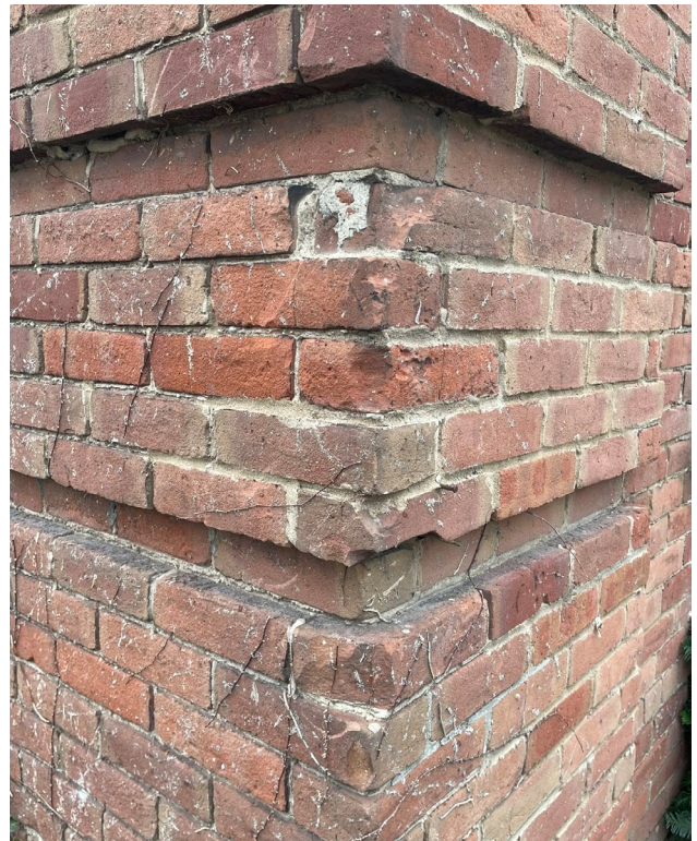
Fig. 5.8. North east corner: example of brick spalling and erosion in limited areas.
