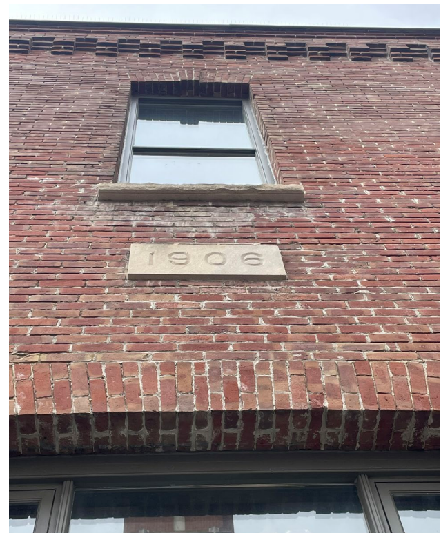
Fig. 5.12. East facade: datestone in good condition and example of mortar repairs and efflorescence under window sill.
