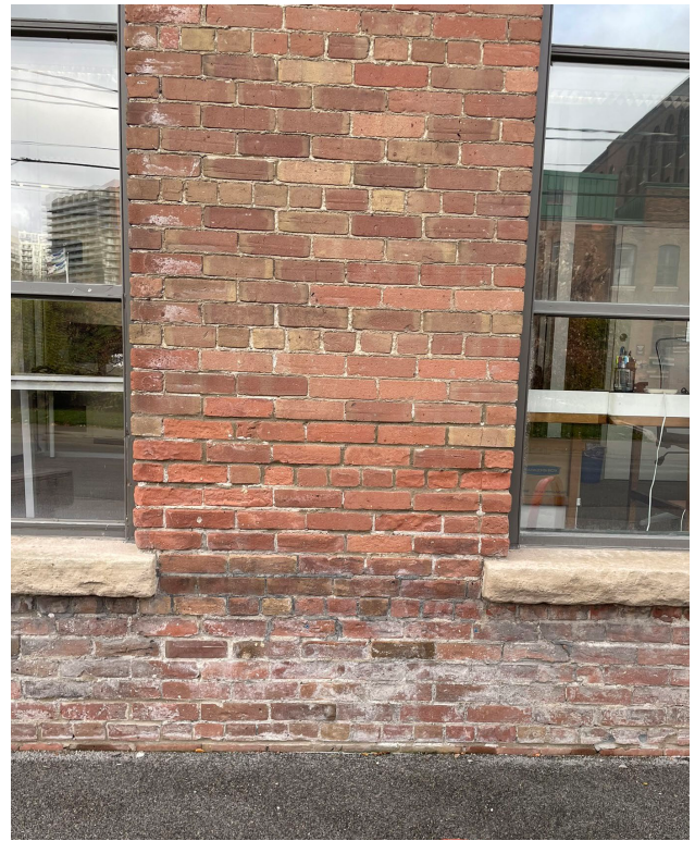
Fig. 5.2. North facade: example of efflorescence, and brick spalling at the building base.
