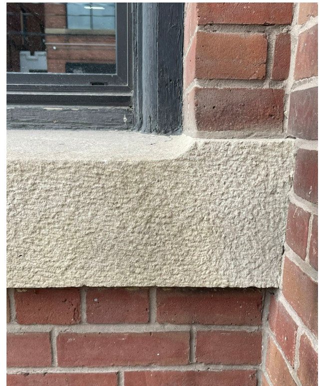
Fig. 5.18. East facade: example of condition of original limestone sills.
