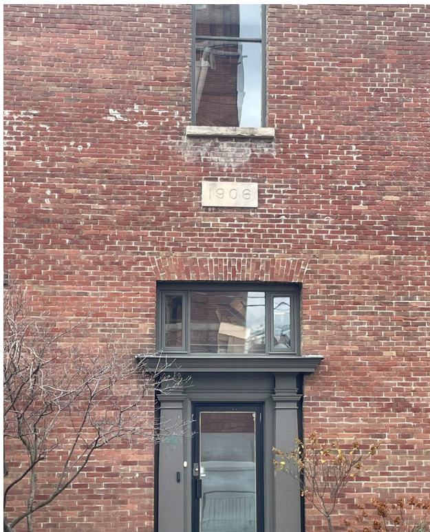
Fig. 5.9. East facade: general brick condition with instances of efflorescence and mortar repairs.
