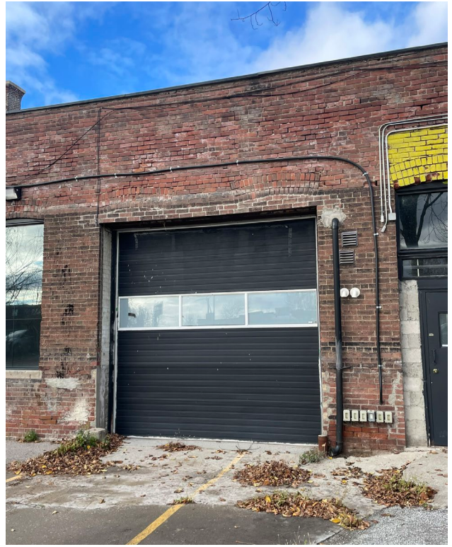
Fig. 5.42. West facade facing the parking lot: masonry in poor condition.
