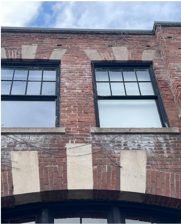
Fig. 5.23. East facade at the second storey addition: example of efflorescence.
