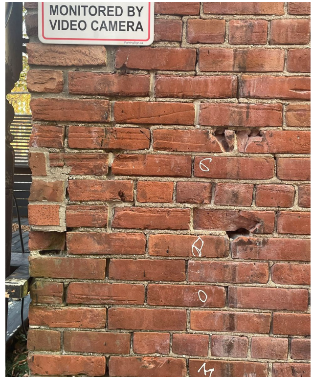
Fig. 5.47. Example of eroding bricks, open joints and incompatible repairs.
