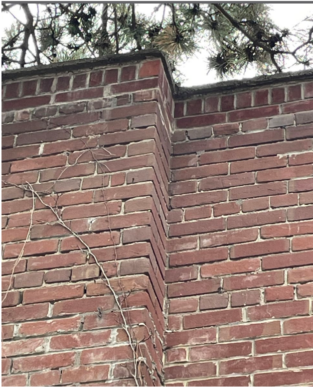
Fig. 5.27. East facade: brick condition at the roof line of the south wing addition.
