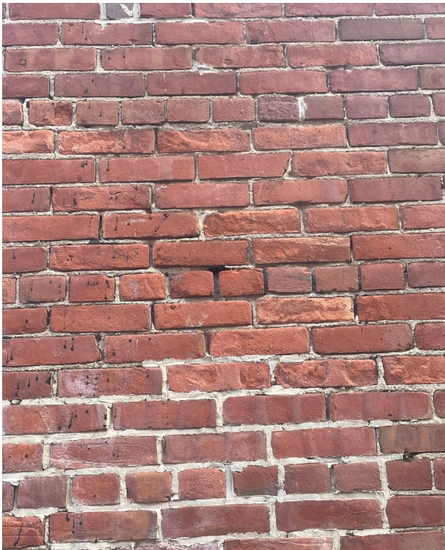
Fig. 5.46. North facade: Example of brick spalling, open joints and incompatible mortar repairs.
