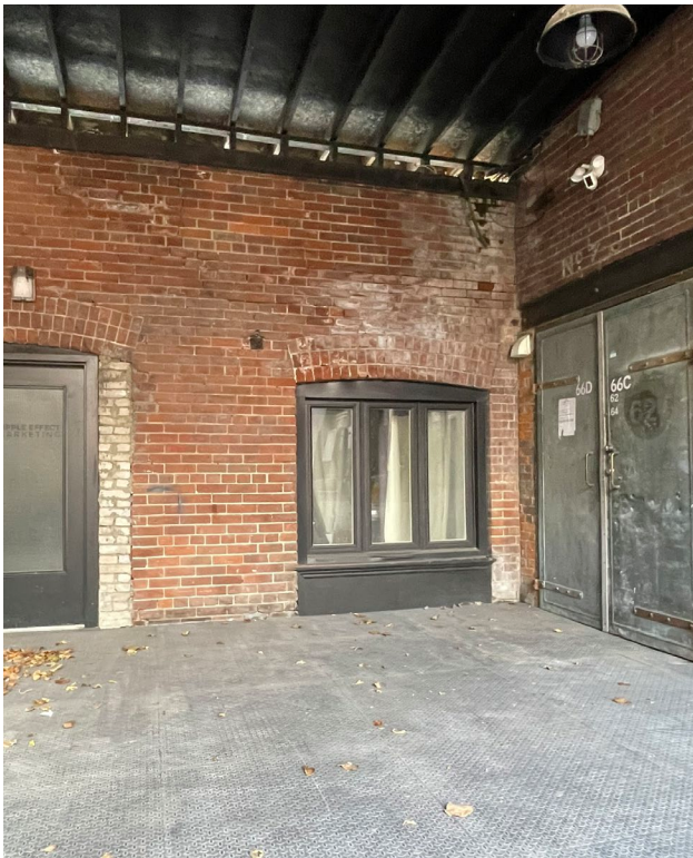
Fig. 5.35. Courtyard: masonry in fair to poor condition.
