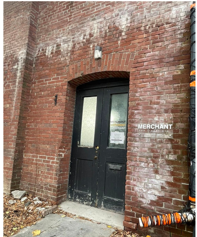
Fig. 5.26. East facade: example of efflorescence at the south wing addition.
