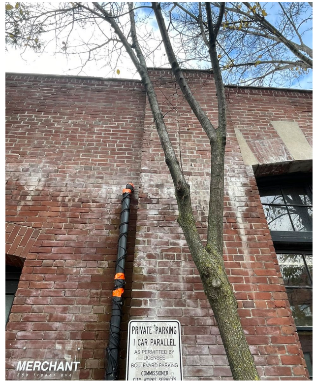
Fig. 5.24. East facade at the second storey addition: example of efflorescence.
