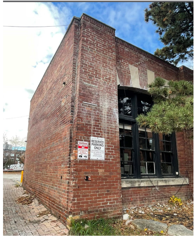
Fig. 5.28. South end of the south wing addition showing florescence, soiling and mortar repairs.
