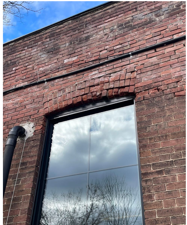
Fig. 5.38. South facade facing the parking lot: masonry in poor condition.
