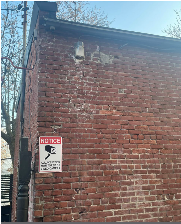
Fig. 5.45. North facade showing significant brick deterioration.
