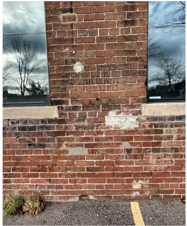
Fig. 5.40. South facade facing the parking lot: example of open joints and mortar repairs.
