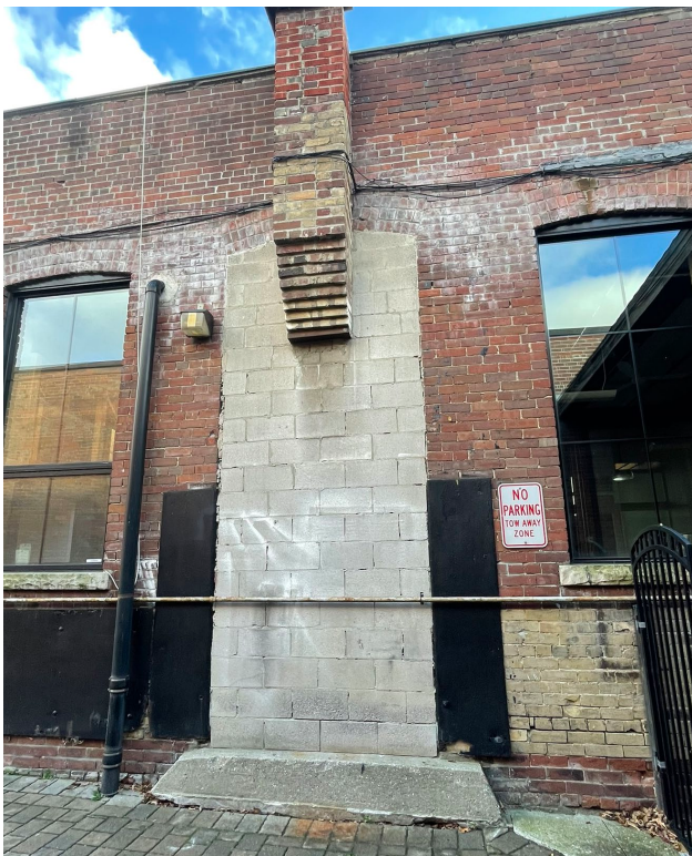
Fig. 5.33. Courtyard: masonry replacements and poor condition in some areas.
