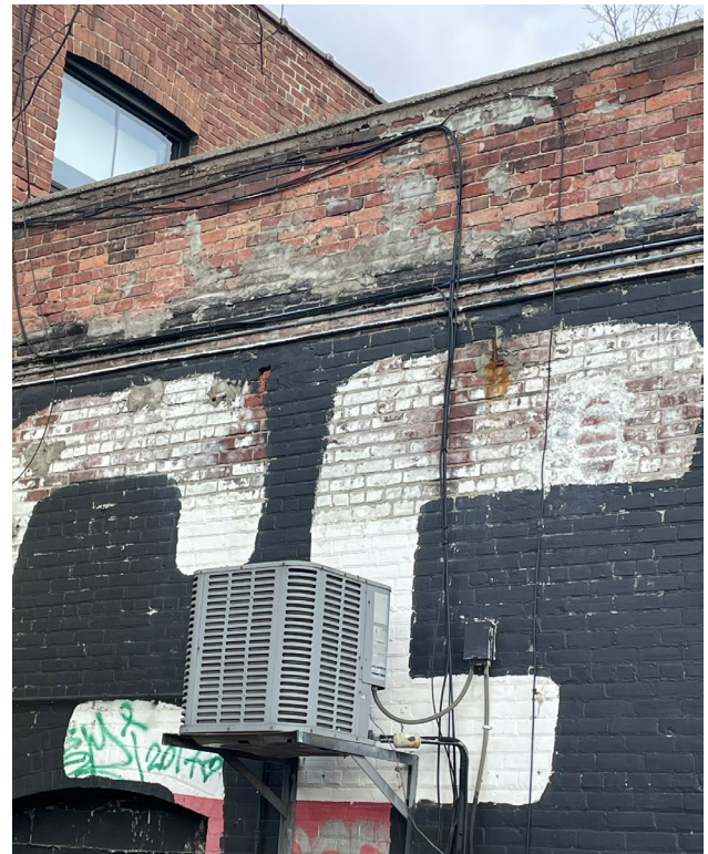
Fig. 5.36. West facade facing the parking lot: masonry in poor condition.
