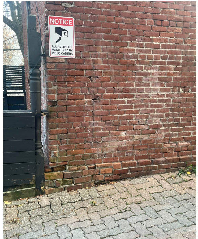
Fig. 5.48. North facade: significant brick deterioration at the corners and lower areas.
