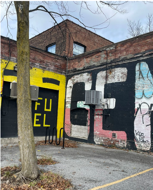
Fig. 5.41. South west corner facing the parking lot: masonry painted and in poor condition in some areas.
