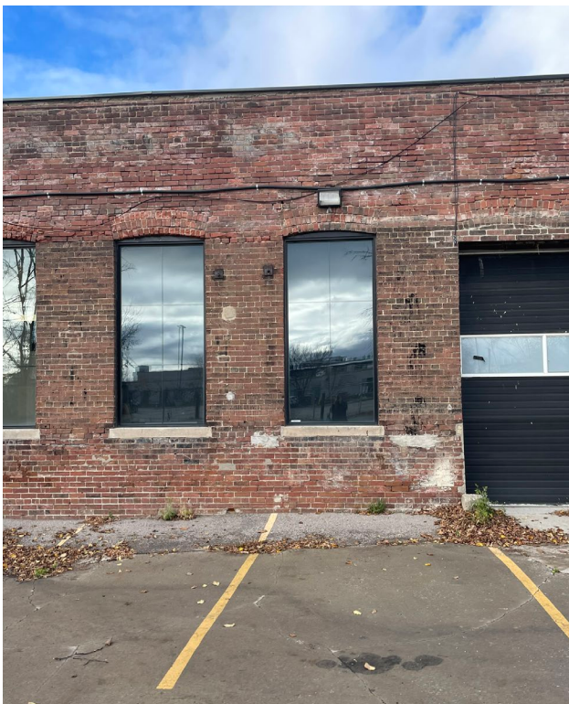
Fig. 5.37. South facade facing the parking lot: masonry in poor condition.
