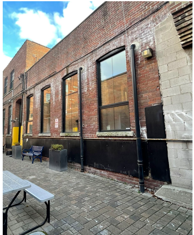
Fig. 5.34. Courtyard: masonry if fair to poor condition, and contemporary window replacements.
