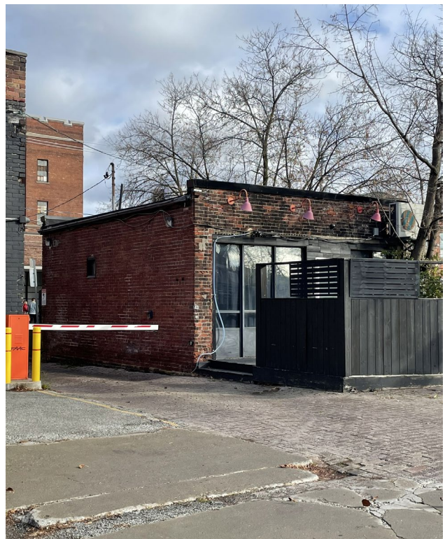
Fig. 5.43. West facade facing the parking lot: masonry in poor condition.
