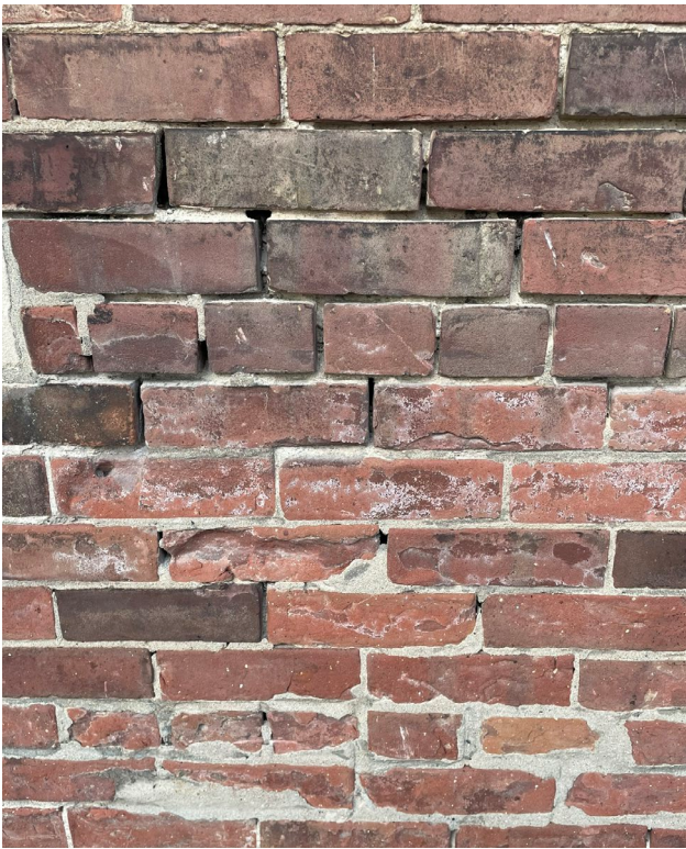
Fig. 5.39. South facade facing the parking lot: example of open joints and mortar repairs.
