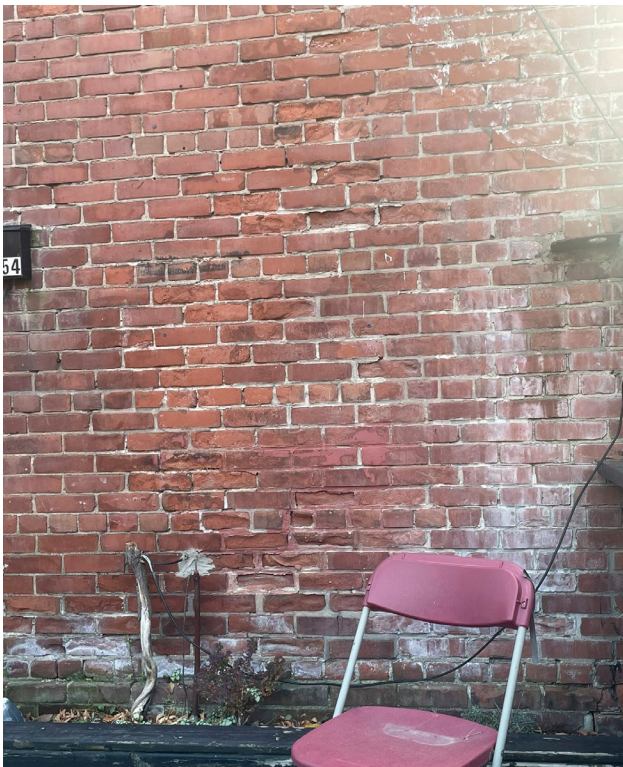
Fig. 5.50. East facade: example of poor brick conditions including spalling, efflorescence, failing mortar joints.
