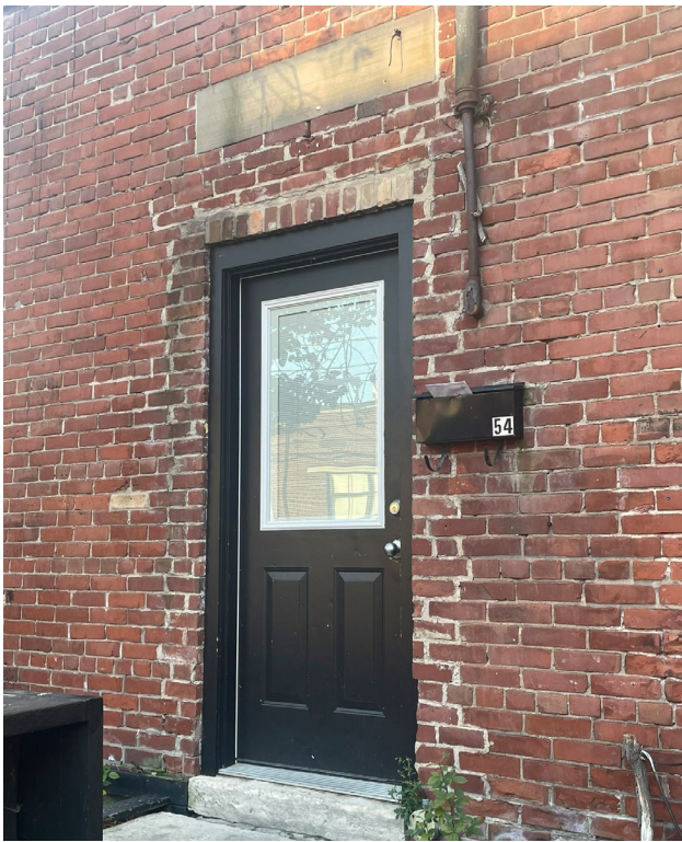
Fig. 5.49. East facade poor mortar repairs at the front door.
