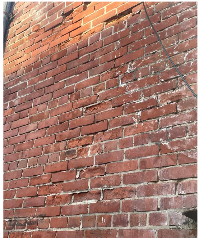
Fig. 5.52. Example of masonry spalling and deterioration.
