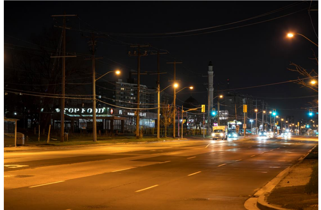
Conventional high-pressure sodium cobra head: Lawrence Avenue East (between Brimley Road & Birchmount Road)
