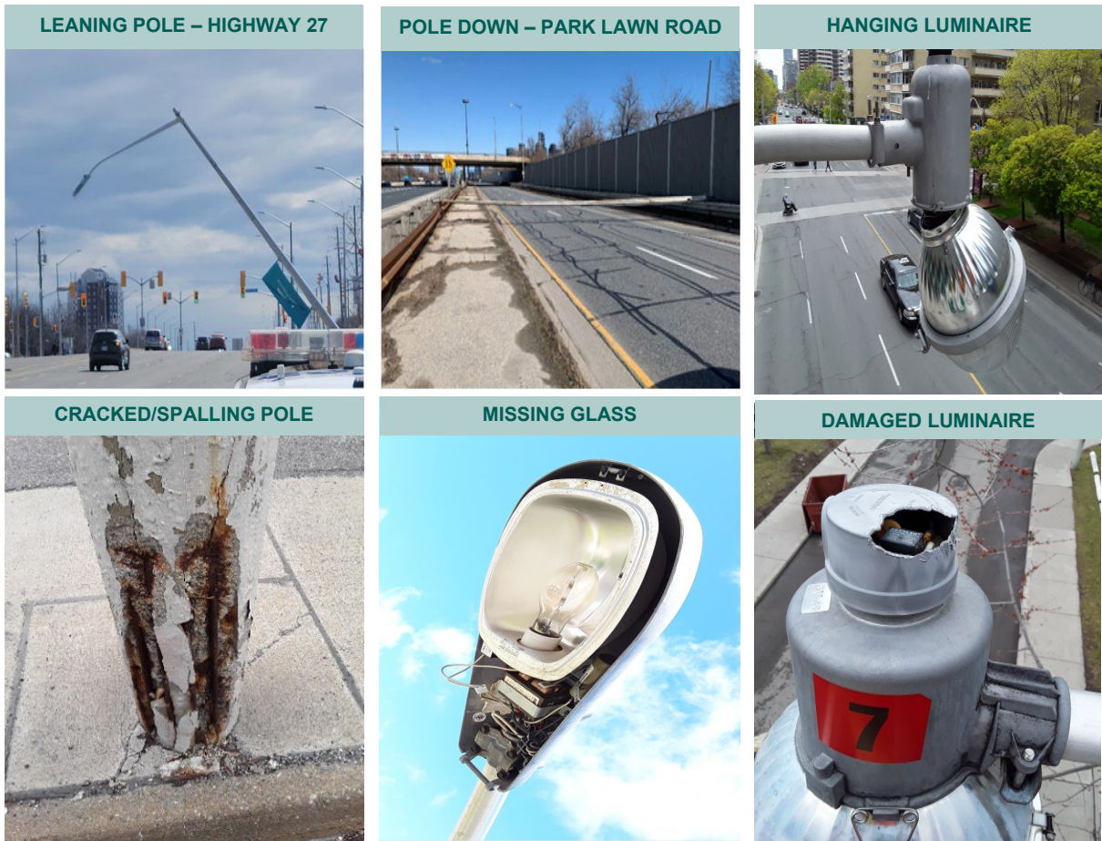
Figure 13: Recent Streetlight Asset Failures
