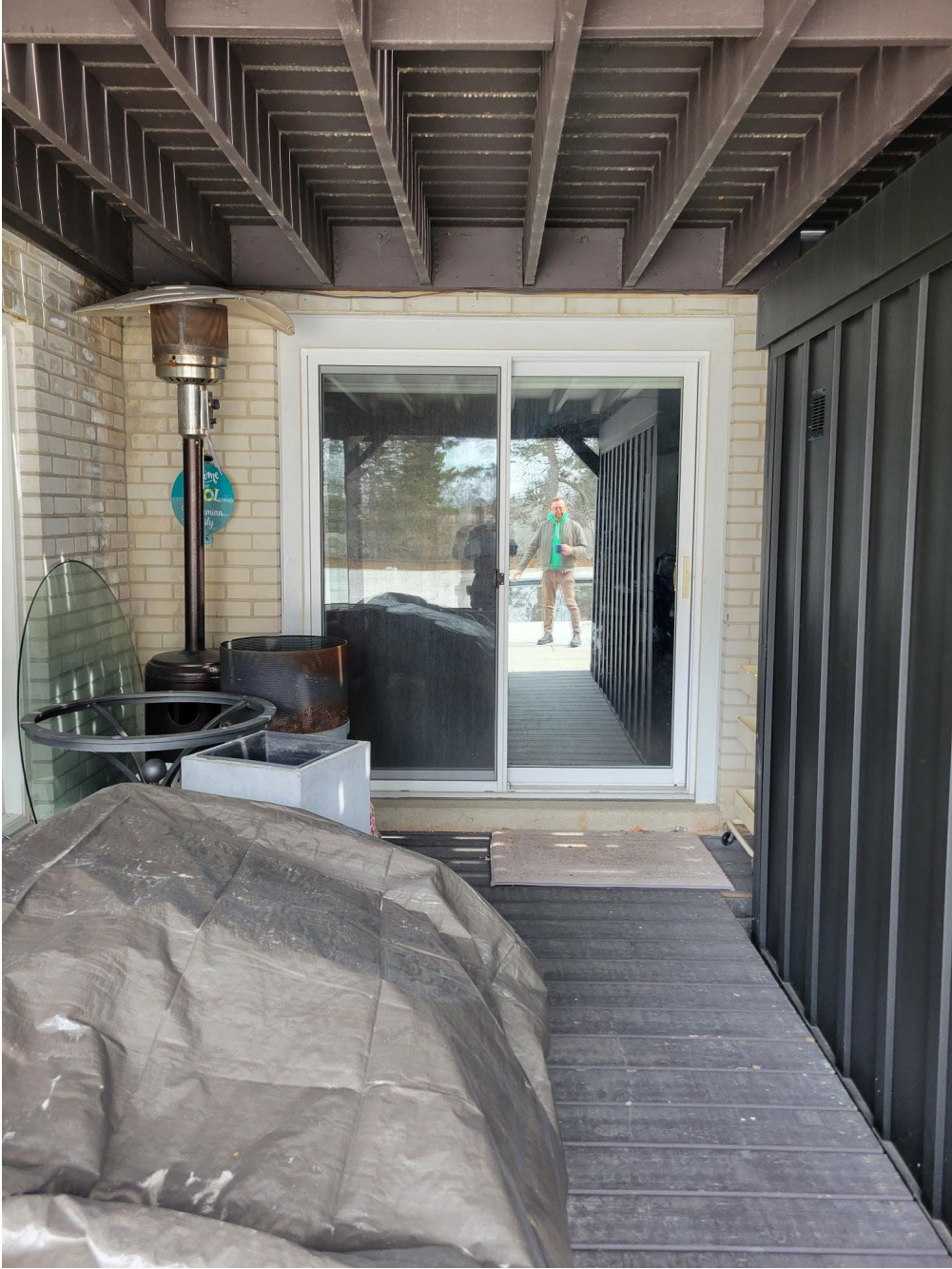
Attachment B: Rear west facing egress from property. Proposed gate location. Taken by Municipal Licensing and Standard Staff.
