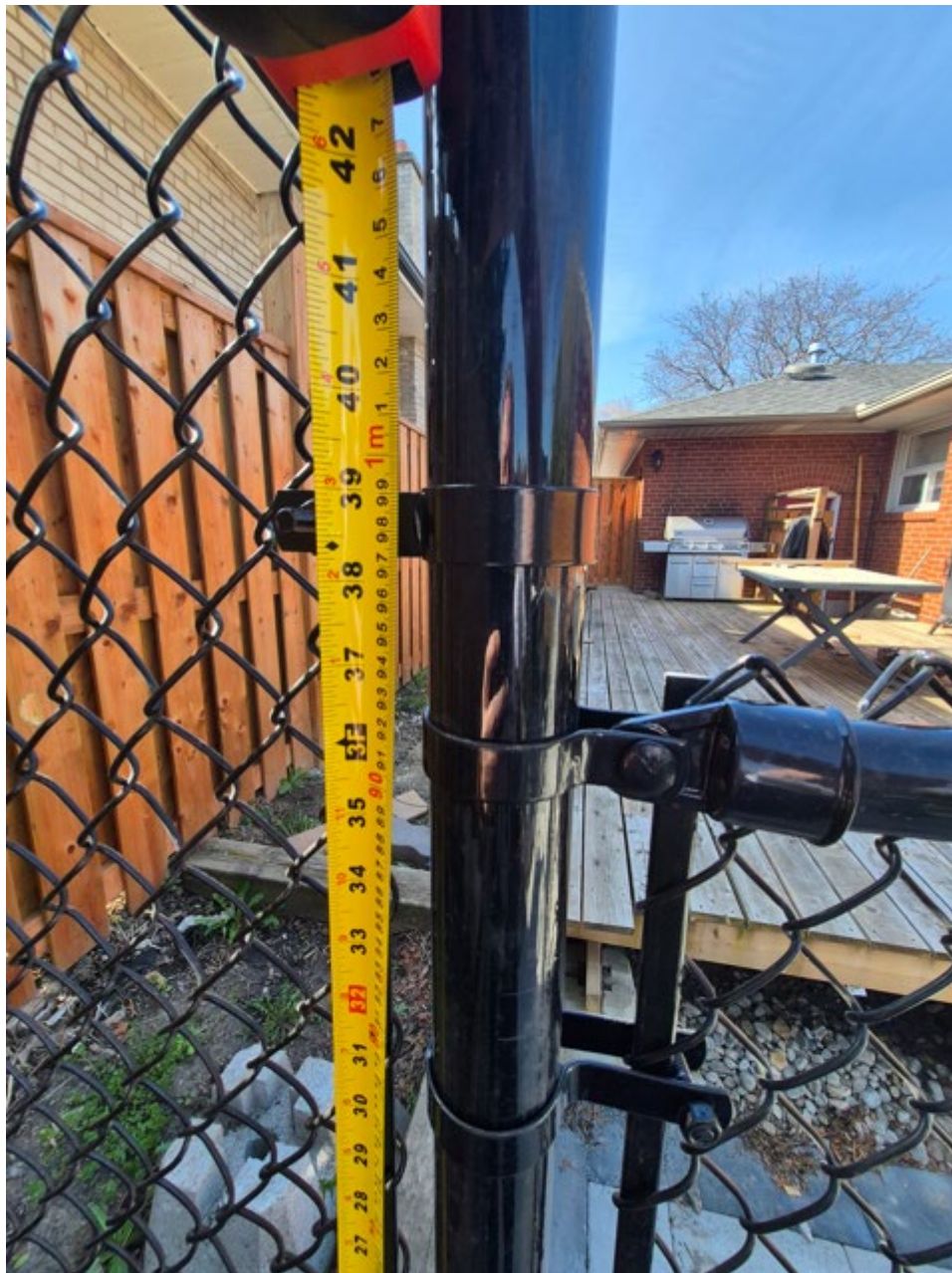
Attachment 4: Officers photo – Fence height, climbable condition
