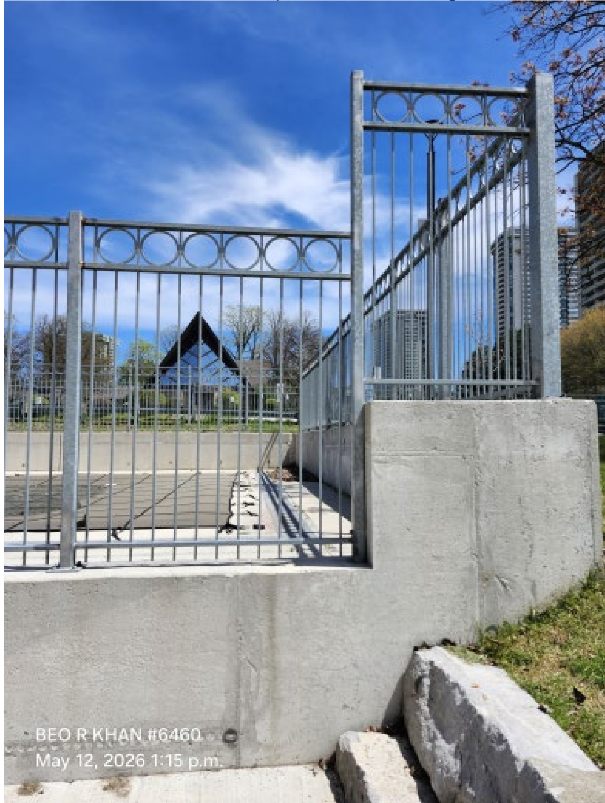
Attachment 2: Attachment 2: Officers photo – Fence below height, climbable condition
