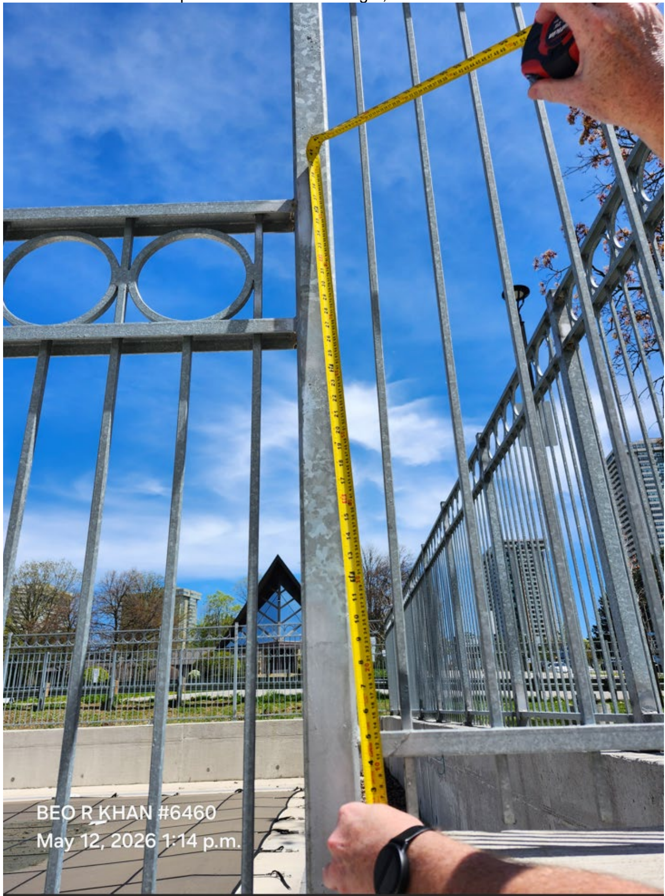
Attachment 4: Officers photo – Fence below height, climbable condition
