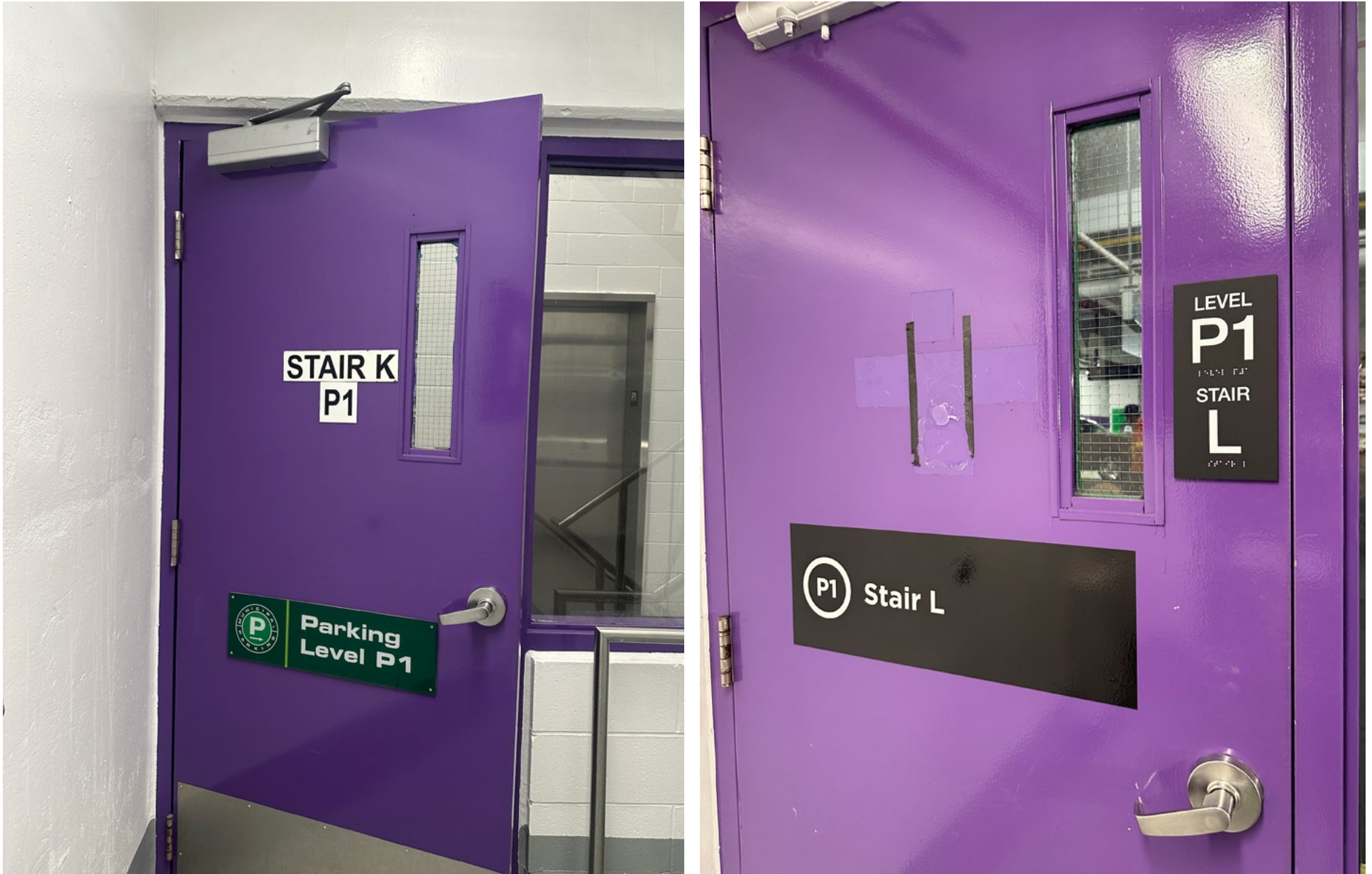
(Above – Figure 5) CP215 before egress stairwell exit with no AODA compliant signage. CP215 after AODA signage upgrades to meet building code compliance, using tactile lettering with low-glare materials, high-contrast colour, and braille.
