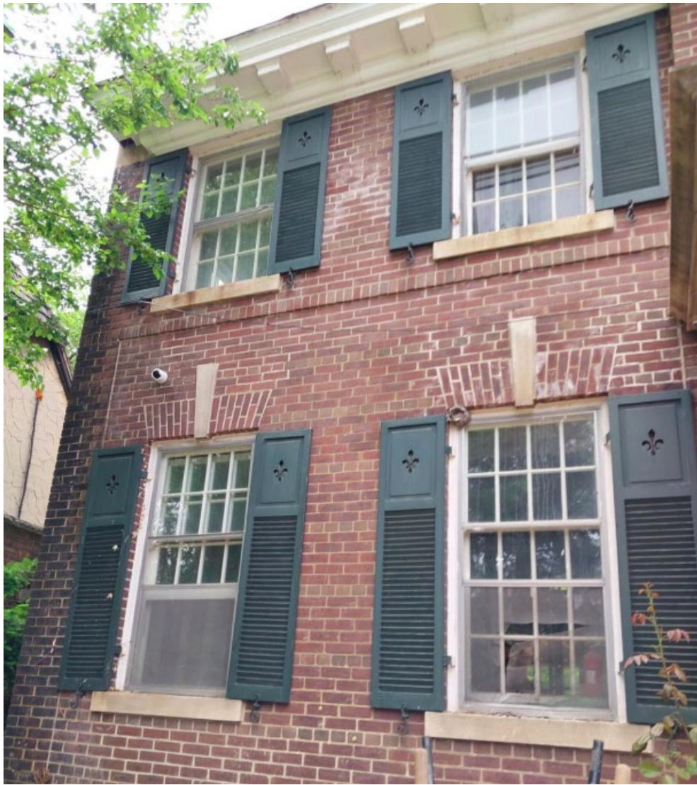
Contextual photo of the existing original windows on the western side of the south elevation.
