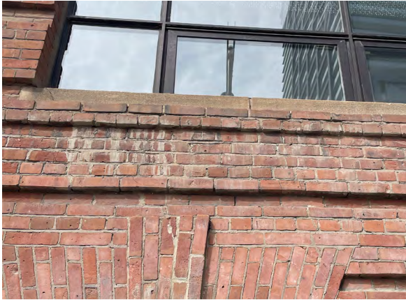
Figure 60. East elevation staining and soiling under sill (ERA, 2022).
