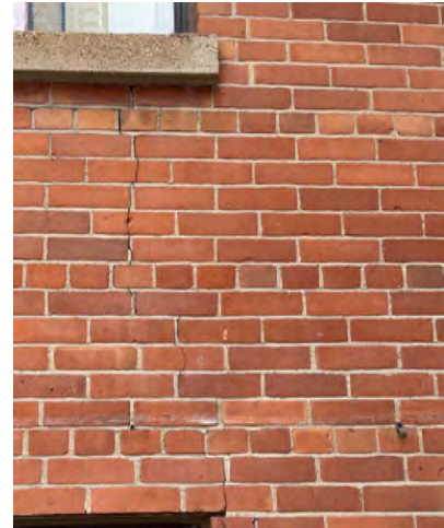
Figure 82. South elevation step cracking (ERA, 2022).
