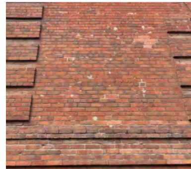
Figure 58. East elevation repair work, soiling and mortar loss (ERA, 2022).
