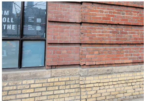
Figure 65. East elevation central bay return displaying change in brick, mortar loss, chipping and cracks (ERA, 2022).
