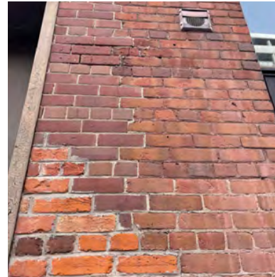
Figure 73. Brick replacement, mortar loss, spalling and repointing on the west elevation (ERA, 2022).
