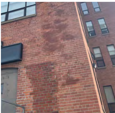
Figure 77. West elevation at east side with moisture staining (ERA, 2022).
