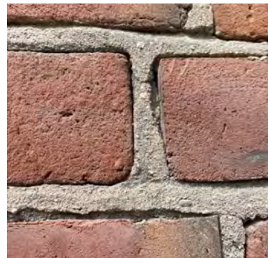
Figure 59. East elevation brick rounding and erosion (ERA, 2022).
