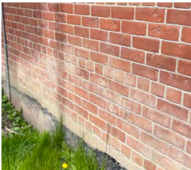
Figure 83. South elevation at grade dust staining and spalling (ERA, 2022).
