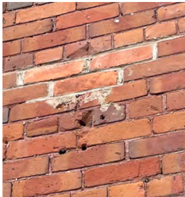
Figure 75. West elevation at second floor with brick replacement, repointing, holes and spalling (ERA, 2022).
