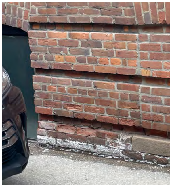
Figure 70. North elevation at grade spalling and efflorescence (ERA, 2022).
