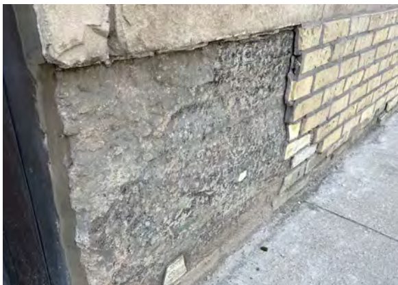
Figure 64. East elevation exposed foundation and loss of brick veneer (ERA, 2022).
