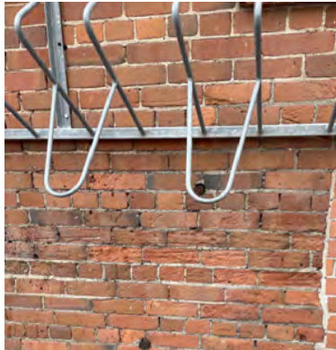
Figure 72. West elevation with mounted bike rack, brick holes, spalling and mortar loss (ERA, 2022).
