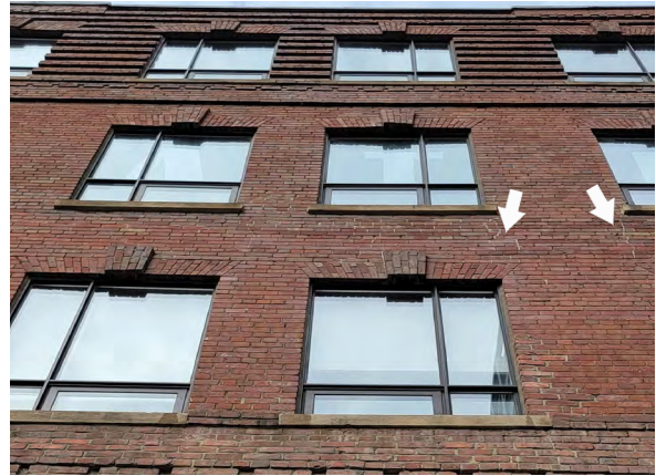
Figure 61. East elevation step cracking (ERA, 2022).
