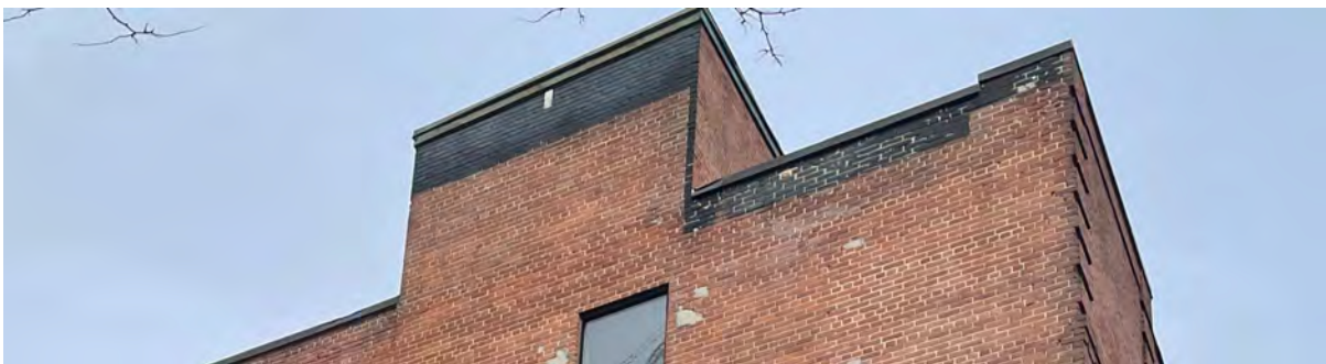
Figure 86. South elevation parapet paint or tar remnants (ERA, 2022).
