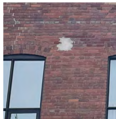
Figure 76. West elevation at second floor with typical parging patch (ERA, 2022).
