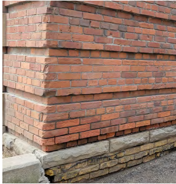
Figure 68. Brick on the North-east corner at grade with breakage, mortar loss, spalling and soiling (ERA, 2022).
