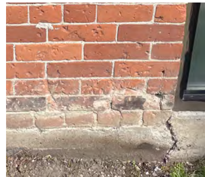
Figure 85. South elevation at grade dust staining and spalling (ERA, 2022).
