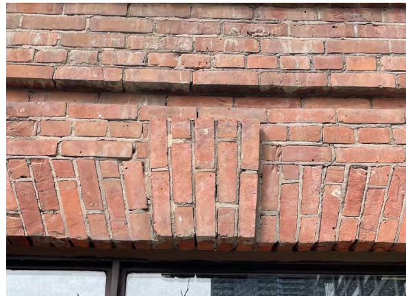
Figure 63. East elevation mortar loss and soiling (ERA, 2022).
