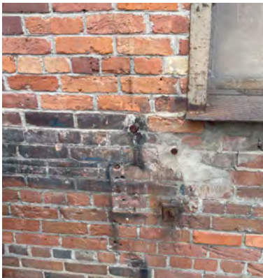
Figure 74. West elevation near grade with staining, brick replacement, parging, holes and repointing (ERA, 2022).
