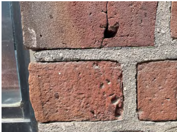
Figure 62. East elevation holes and erosion of brick (ERA, 2022).
