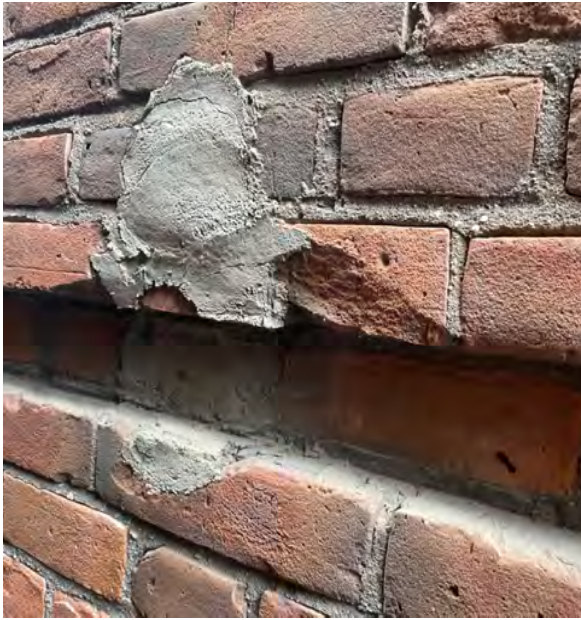
Figure 67. Brick on the north elevation near grade with parging and breakage (ERA, 2022).
