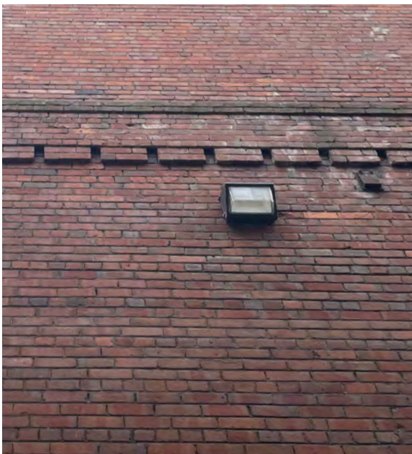
Figure 69. North elevation, second floor banding with mortar loss, spalling and soiling (ERA, 2022).
